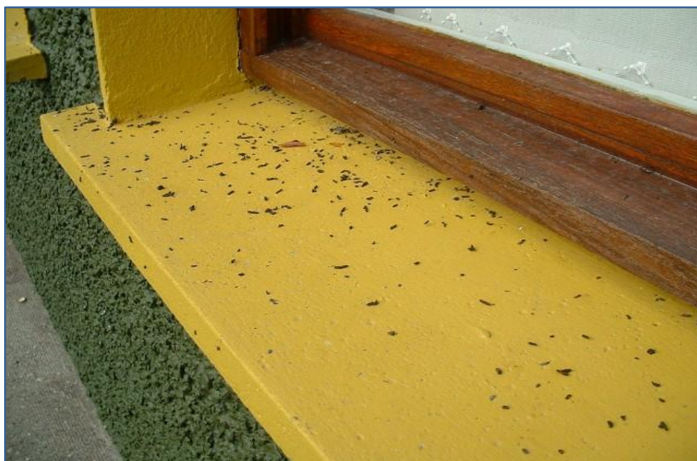
Figure 15 Pipistrelle droppings on window sill beneath roost access point.
