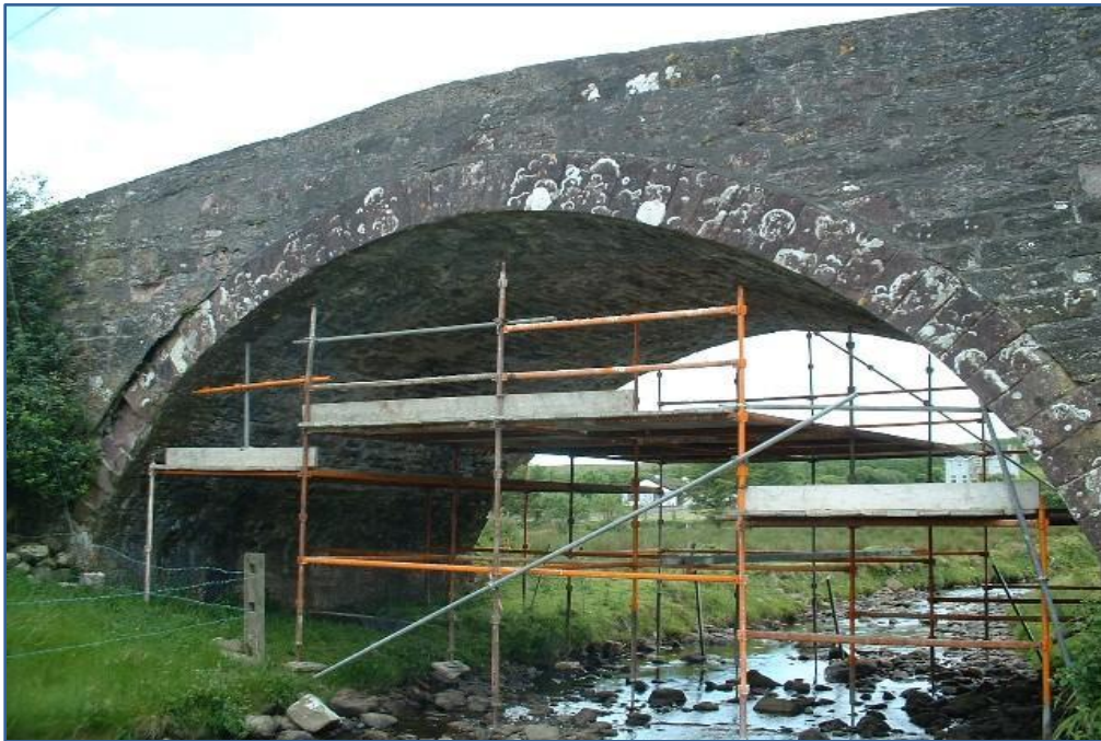
Figure 16 Bridge repair works which may impact bat roosting sites. [Photograph: Conor Kelleher]
