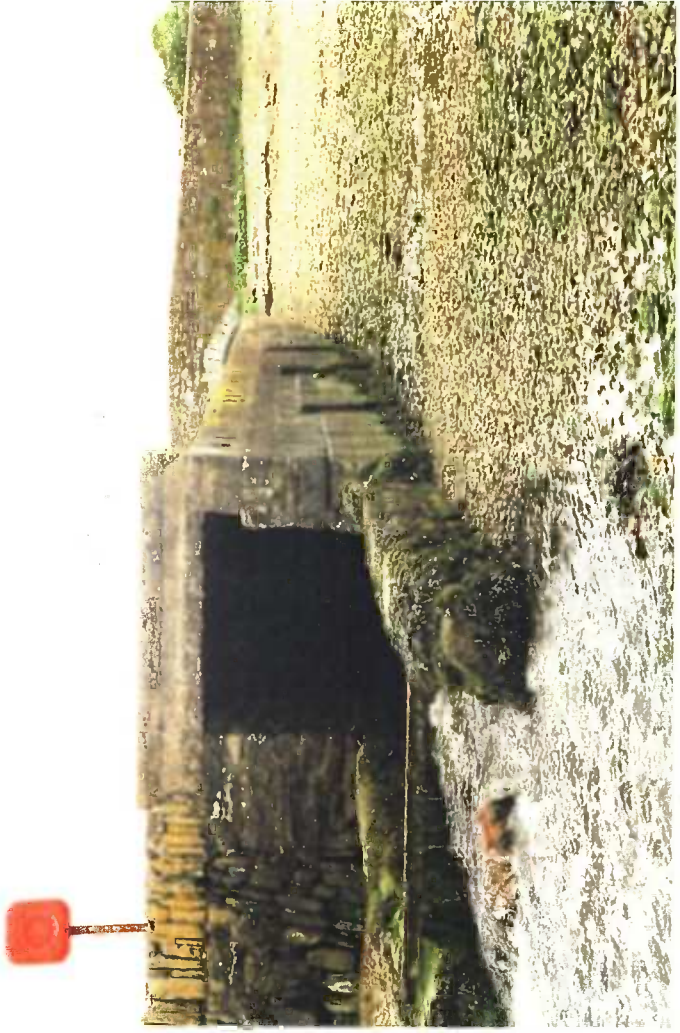
Cuskinny Lake. Water flowing from outlet channel onto the beach.
