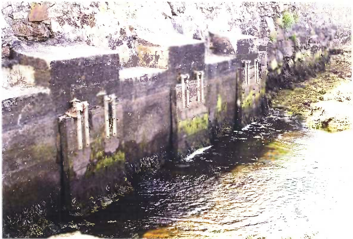
Moorlagh Lough. Sluice gates on the seaward side of the causeway.
