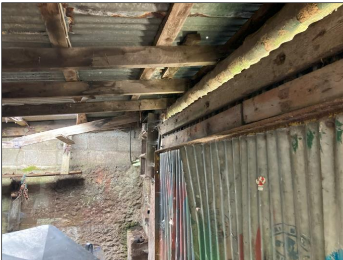
Plate 8 Interior of Shed 1 - a few bat droppings were found within. Note the arrangement of roof timbers and paucity of good bat roosts. Some of the roof covering is also missing.
