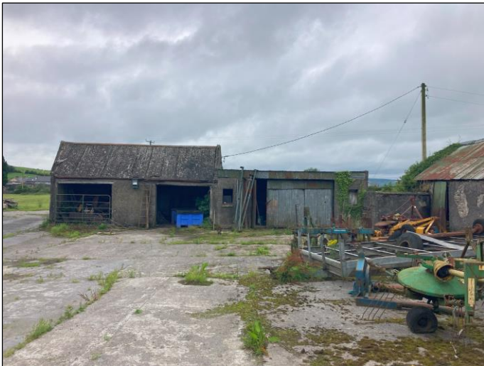
Plate 5 Front of Shed 1 - shed to the right with galvanised metal door - bat droppings present.
