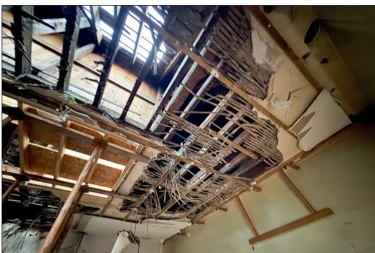
Plate 9 The internal areas of St. Joseph's house could not be inspected due to health and safety issues. However, it was confirmed that the building had been damaged by fire, and internal works had been completed (cleaning out etc.).
