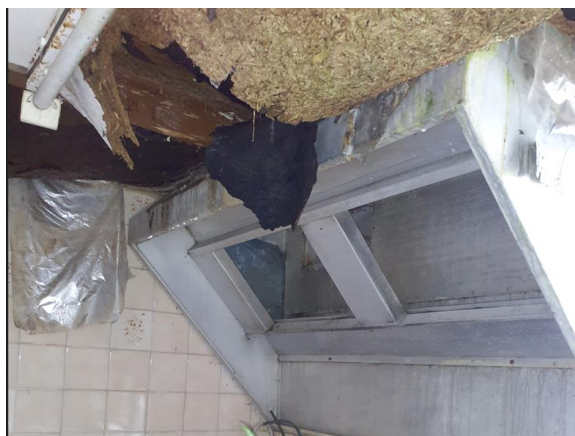
Plate 3. Water damage in ceiling
