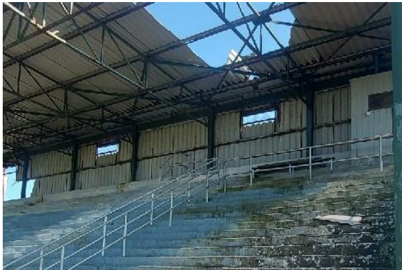
Plate 5. Roof damaged and partially missing
