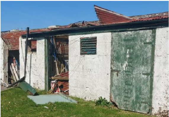
Plate 6. Roof damaged and partially missing
