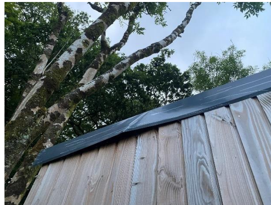
Plate 3-3 Lifting trim on wooden shed
