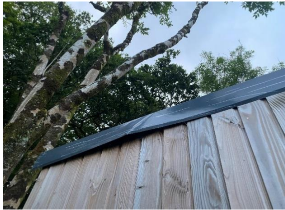
Plate 4 Lifting trim on wooden shed
