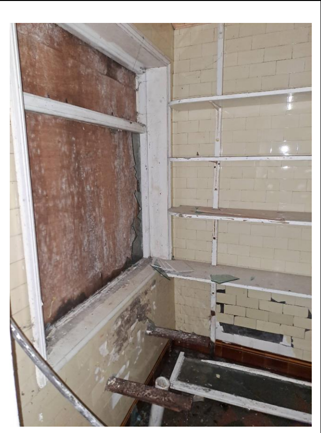
Photo 7: Tiles Damaged in Storeroom
