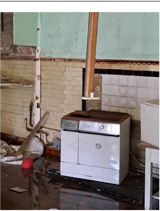
Photo 6: Tiles Bulging Away from Wall
