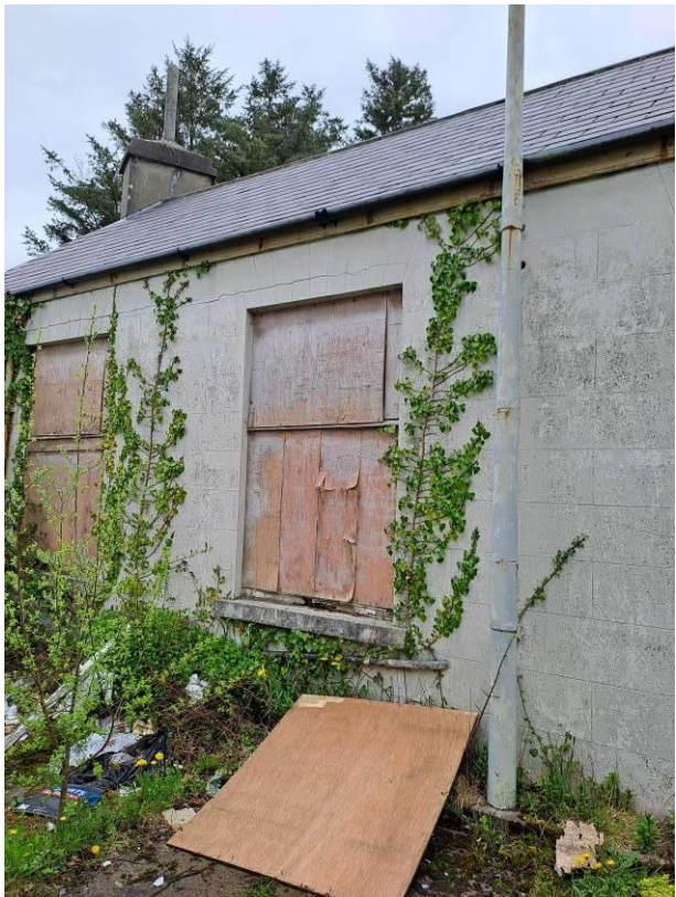
Photo 2: Windows boarded Up
