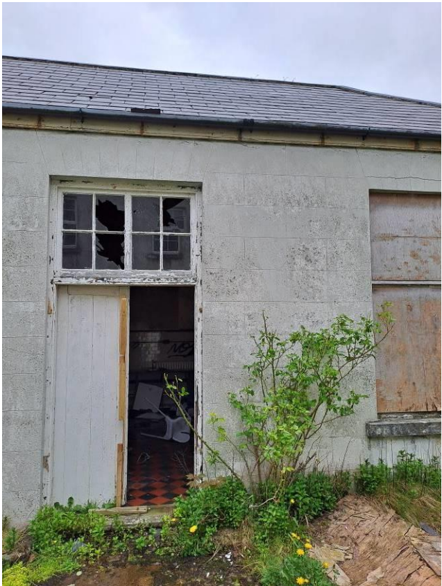
Photo 3: Main Entrance Door Damaged
