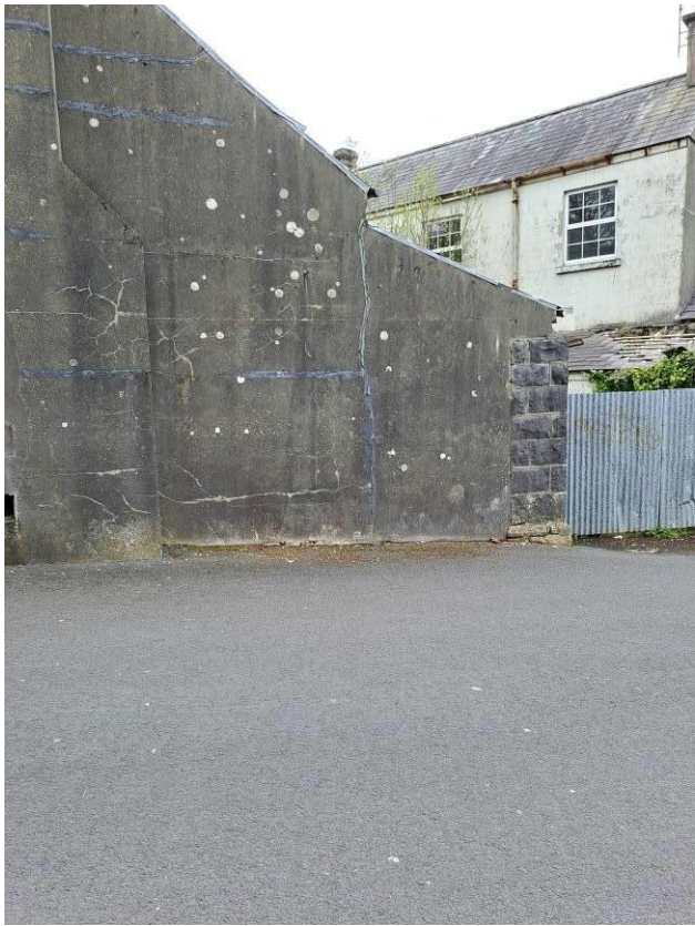
Photo 9: External Plaster in Poor Condition
