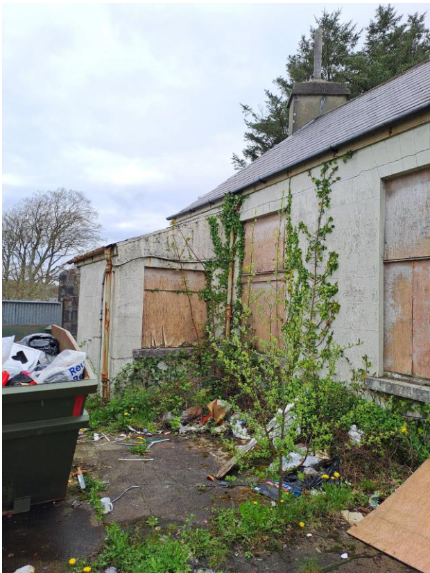
Photo 1: Ivy on External Walls
