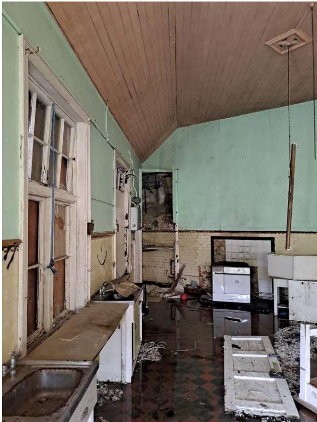
Photo 4: Flooding in Kitchen and Store Area
