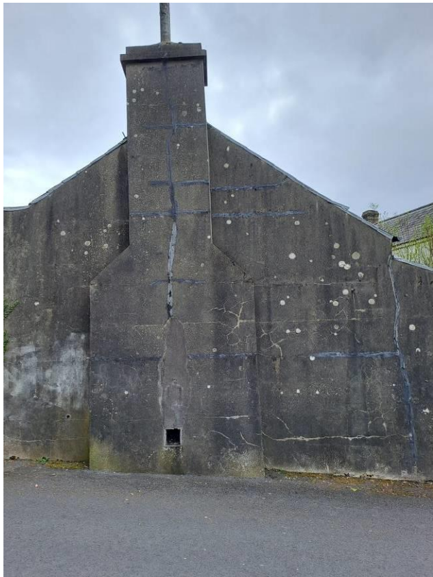
Photo 10: Chimney Stack Plaster Cracking
