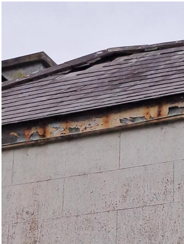
Photo 15: Hole in Roof Structure
