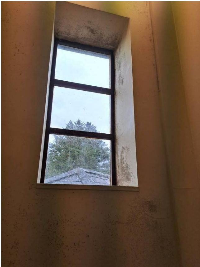
Photo 9: Mould Growth on Internal Wall
