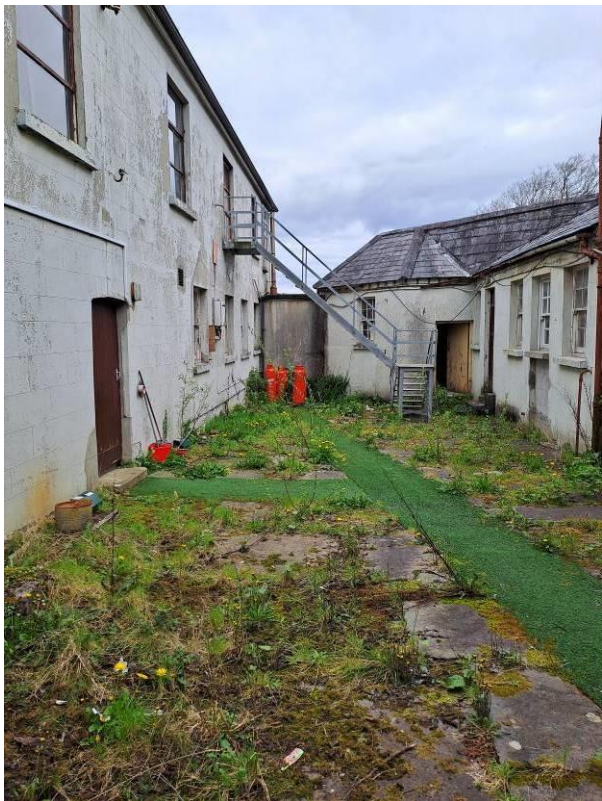
Photo 11: Courtyard in Poor Condition
