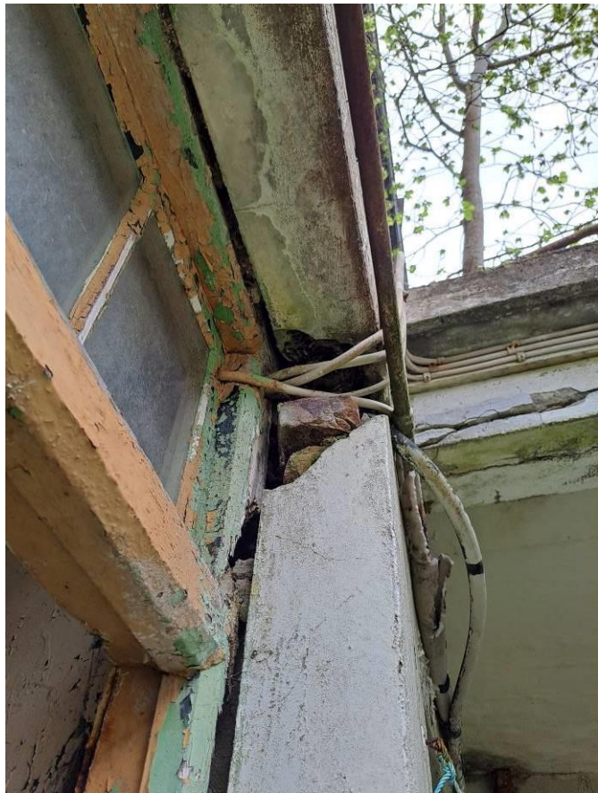
Photo 14: Plaster Damage around Door Reveal
