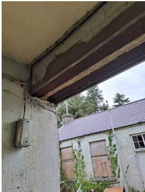
Photo 16: Beams Carrying Building Severely
