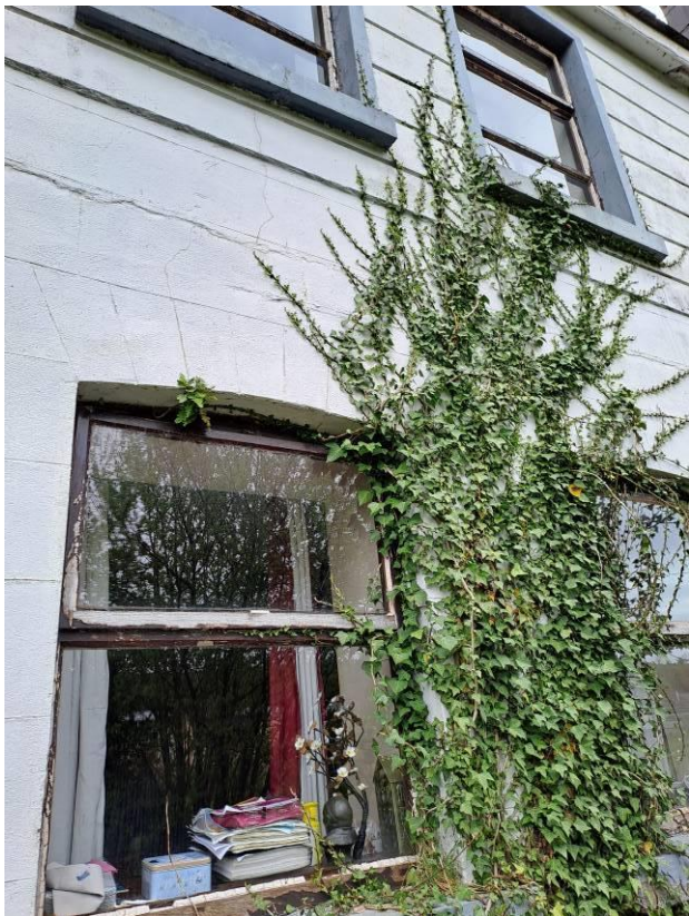
Photo 5: Ivy on External Wall
