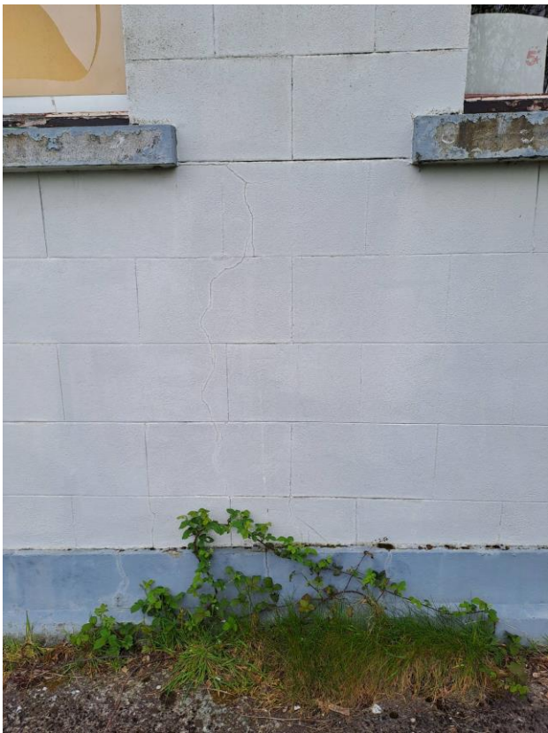
Photo 3: Surface Cracking to Plaster
