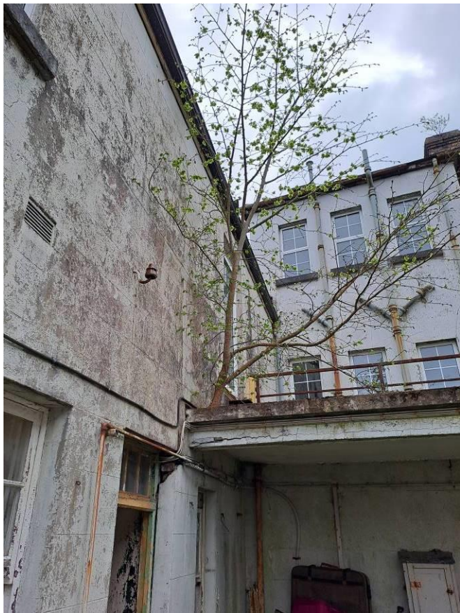
Photo 13: Tree Growing from Flat Roof / Shelter
