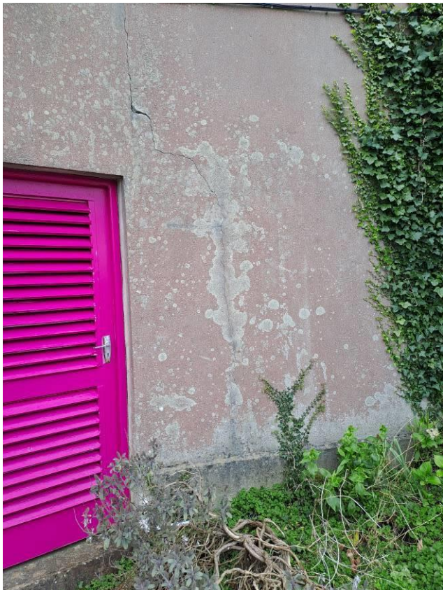
Photo 8: Cracking to Plaster
