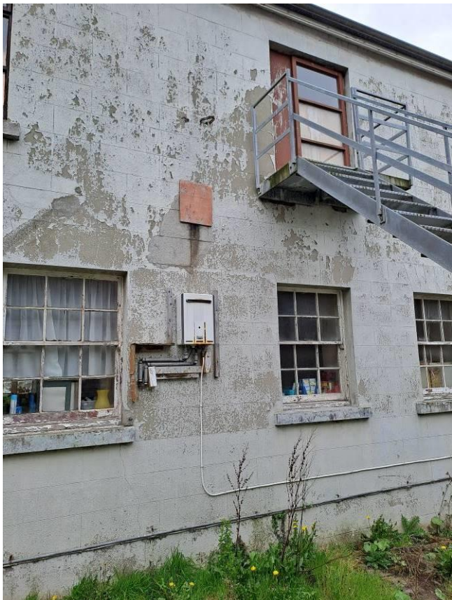
Photo 10: Wall Finishes in Poor Condition
