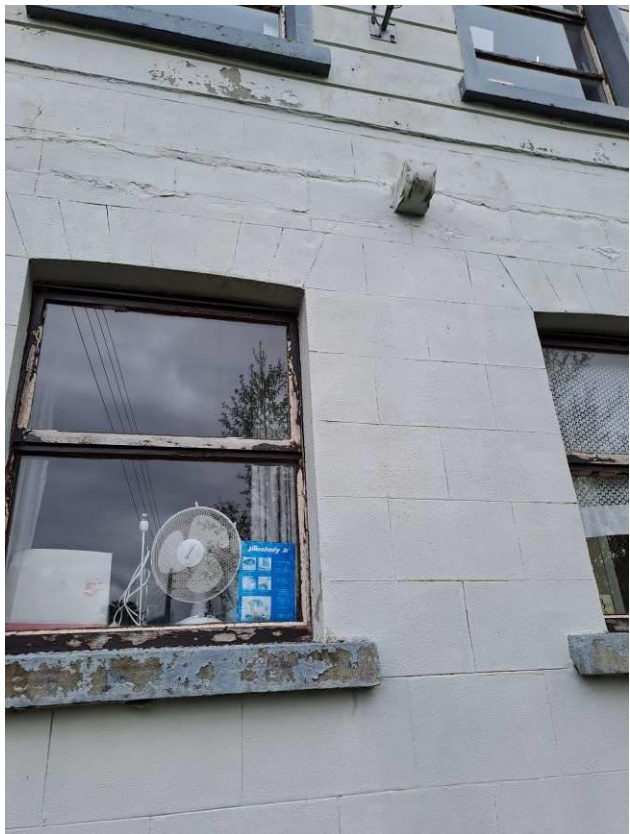
Photo 4: Plaster in Poor Condition
