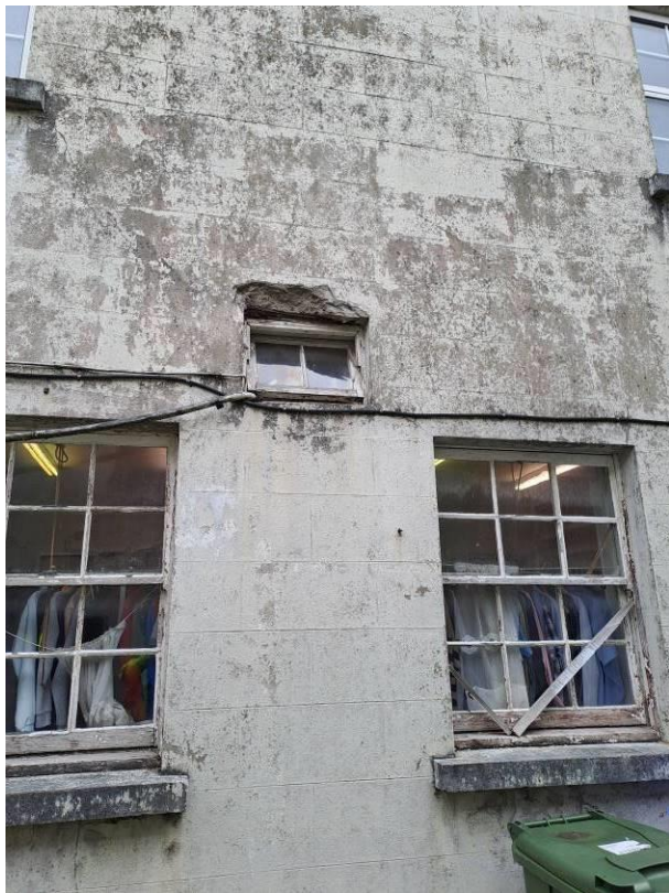
Photo 12: Broken / Damaged Lintel over Window
