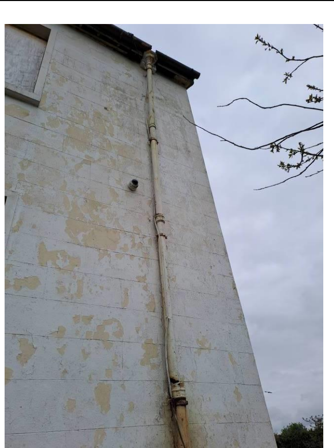
Photo 4: Downpipe Rusted and Broken
