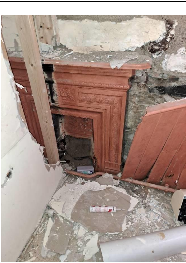
Photo 18: Fireplace Closed Off with Internal Partitions
