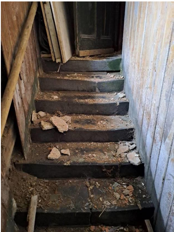
Photo 16: Staircase to Basement Level in Poor Condition
