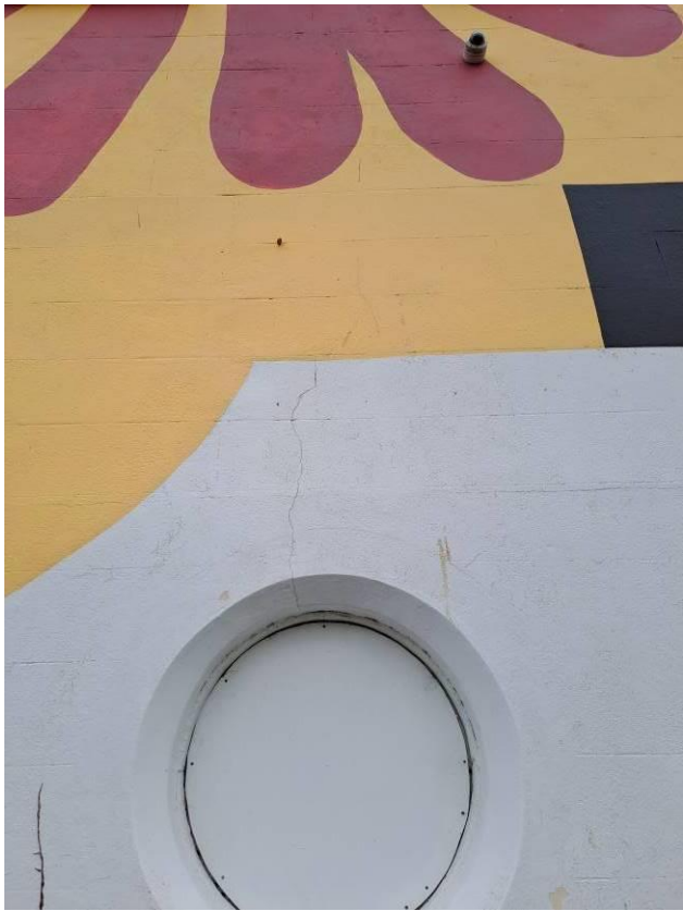
Photo 5: Cracking to Plaster
