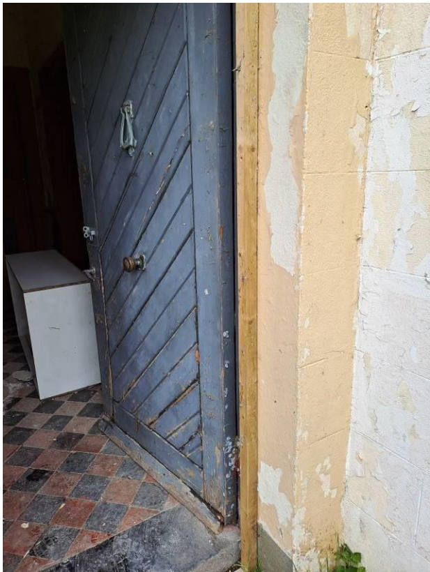
Photo 12: External Door Showing Wear and Tear
