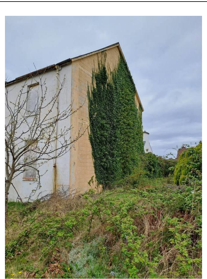
Photo 1: Ivy on External Wall
