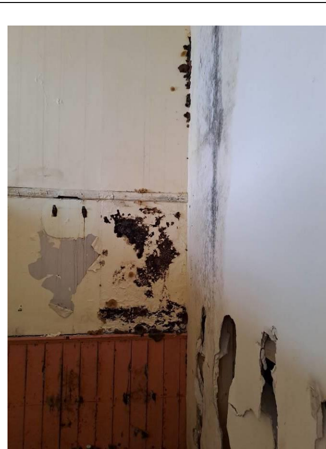
Photo 17: Mould Growth Noted
