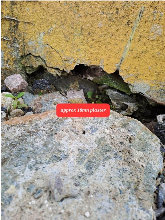
Photo 8: Plaster Cracked / Broken
