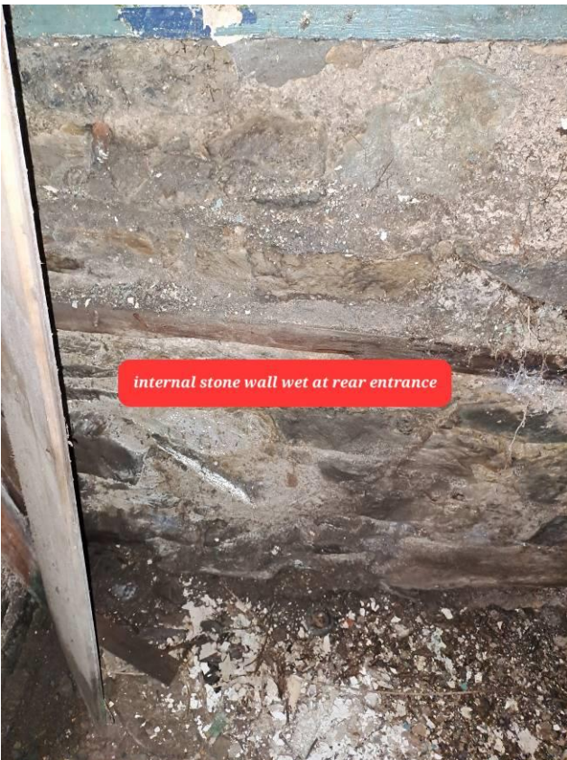
Photo 15: Internal Walls Wet – Moisture Ingress
