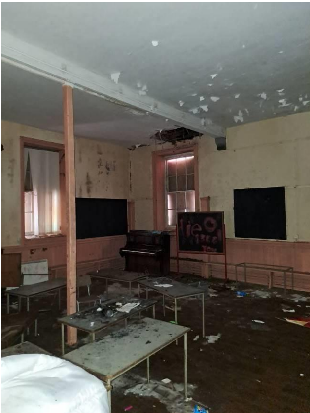
Photo 22: Ceiling in Poor Condition – Hole in Ceiling Noted
