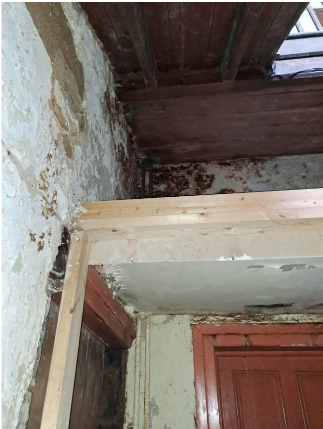
Photo 14: Mould Growing on Internal Walls
