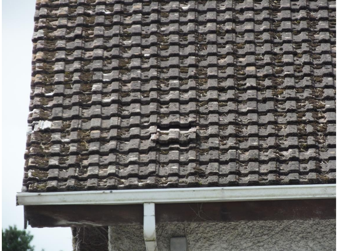
The damaged structure 1
