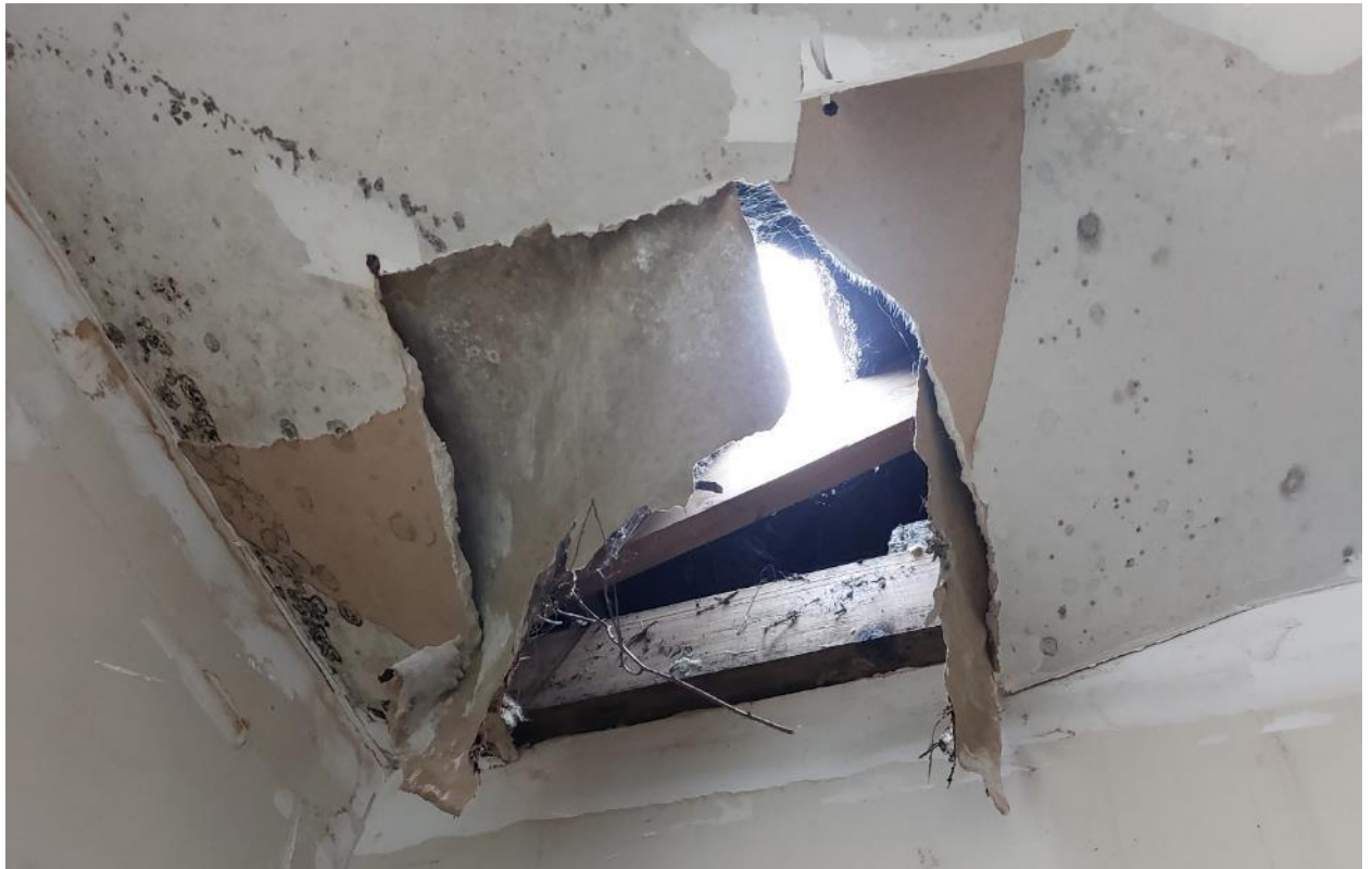
Plate 17: Fallen ceiling of office 7 (1)
