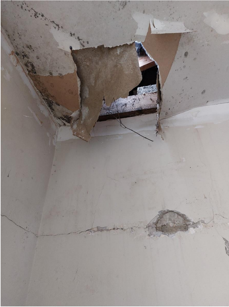
Ceiling of ESB office in question
