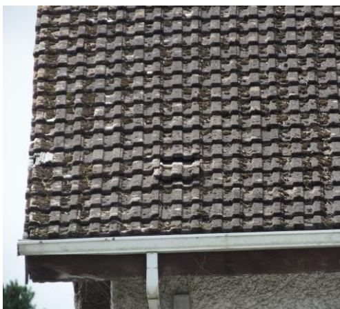
Current ESB roof damage, good candidate for bat tile |
