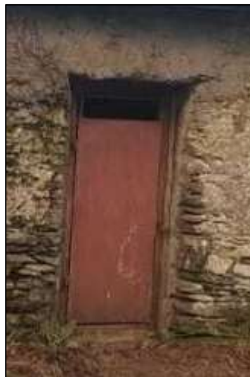
Photo 6: Example of a metal door with letterbox opening (Curraglass SAC roost)
