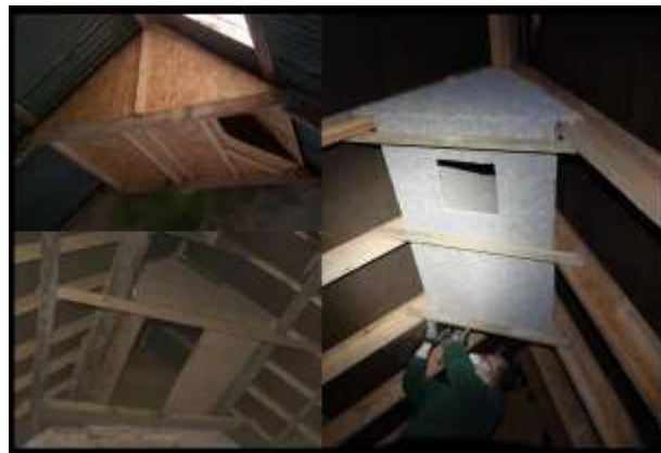
Photo 7: Hot boxes' of various design, installed into roof apex 5
