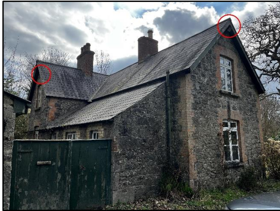
Plate 1: Head Gardener's Cottage roost entrance locations. North-facing gable (left circle) 1 no. soprano observed emerging from soffit. West-facing first-floor window (right circle) with small accumulations of droppings; while no emergence was recorded here, a potential emergence point above the window is circled (See Plate 3).
