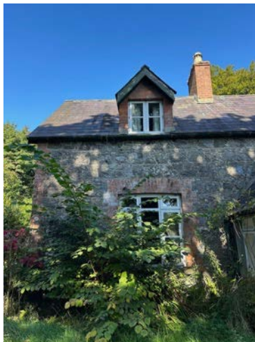
CRACK OVER WINDOW HEAD
