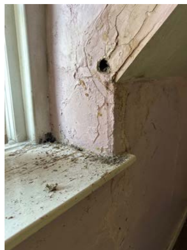
POSSIBLE ROT TO JOIST ENDS
