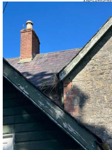
MISSING GUTTER TO GABLE
