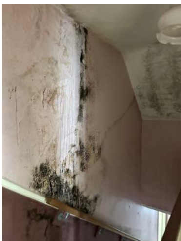
DAMPNESS OVER STAIRS
