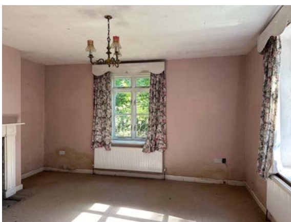
VIEW OF DAMP AT SKIRTING LEVEL TO LIVING ROOM
