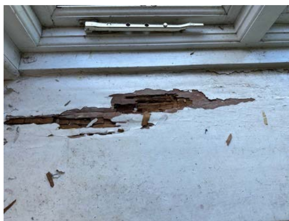
DRY ROT TO WINDOW BOARD
