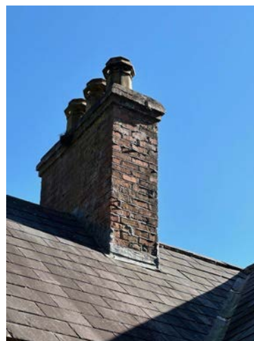
REPOINTING NEEDED TO CHIMNEY
