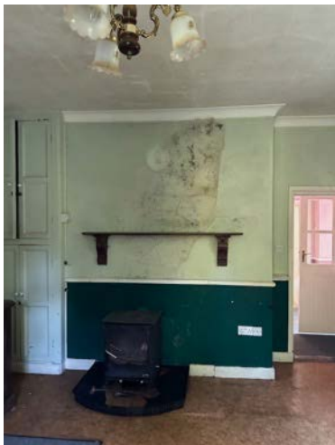
DAMPNESS AT FLUE
