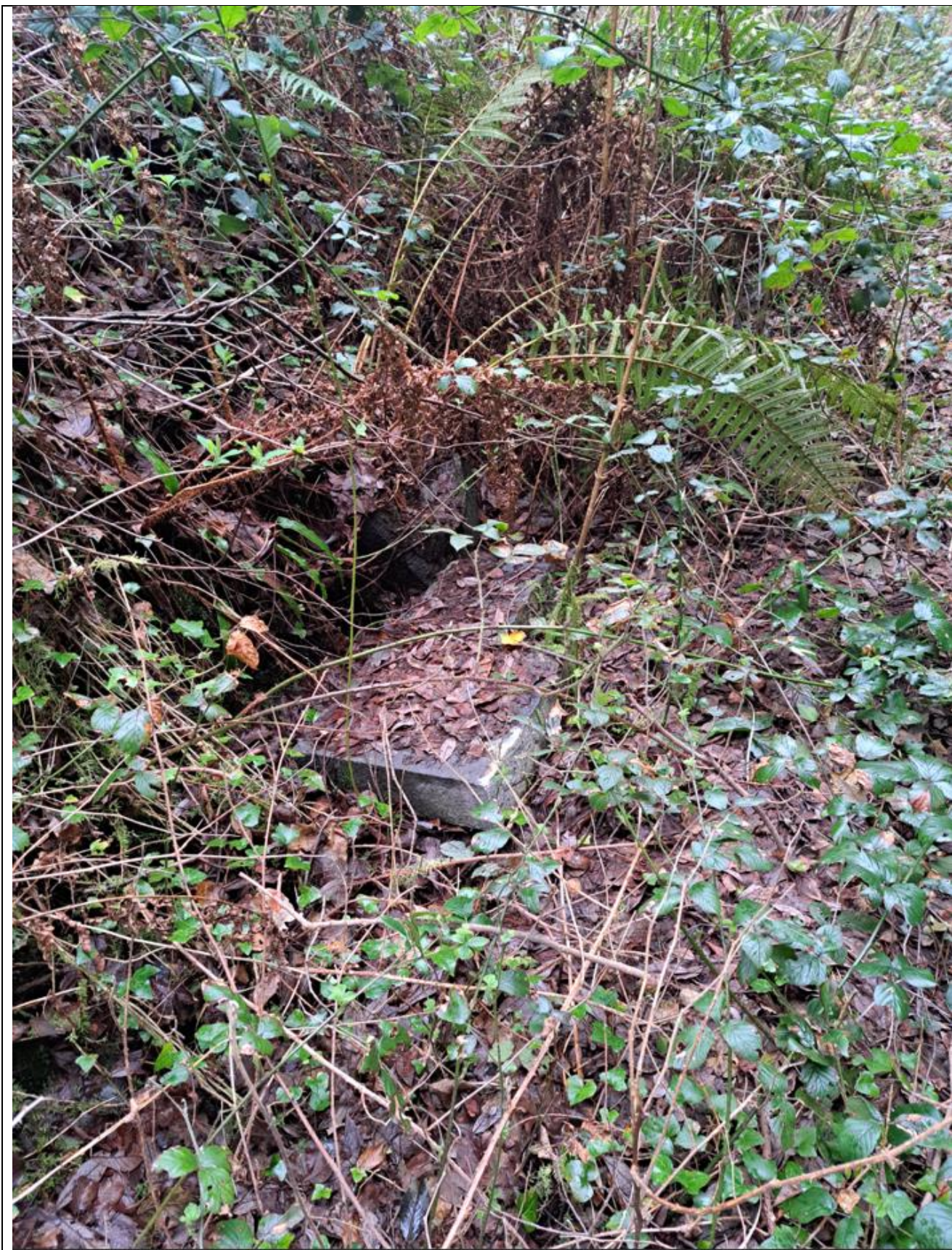
Chimney Works – Remove and replace limestone chimney capping. Some of the stone capping appears to have fallen onto the ground. Provide for new galvanized steel cowls into the chimney pots.
