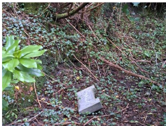
Plate 6 Fallen chimney capping at rear of courthouse.
