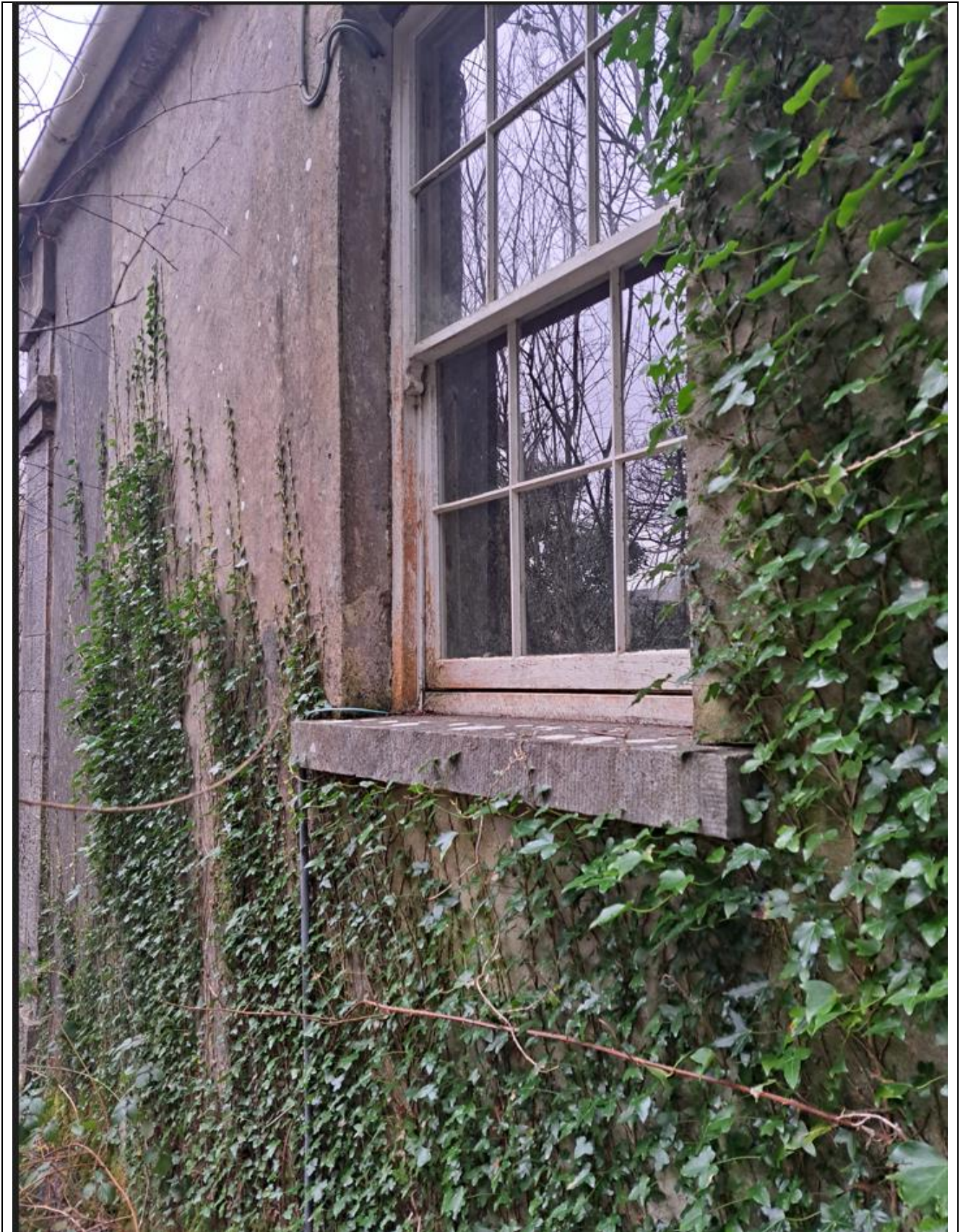
Three number external windows to be sanded, primed and apply two coats of weather proof paint. Replace all ironmongery to bring windows back into use. Include for replacement of one broken single panel of glass
