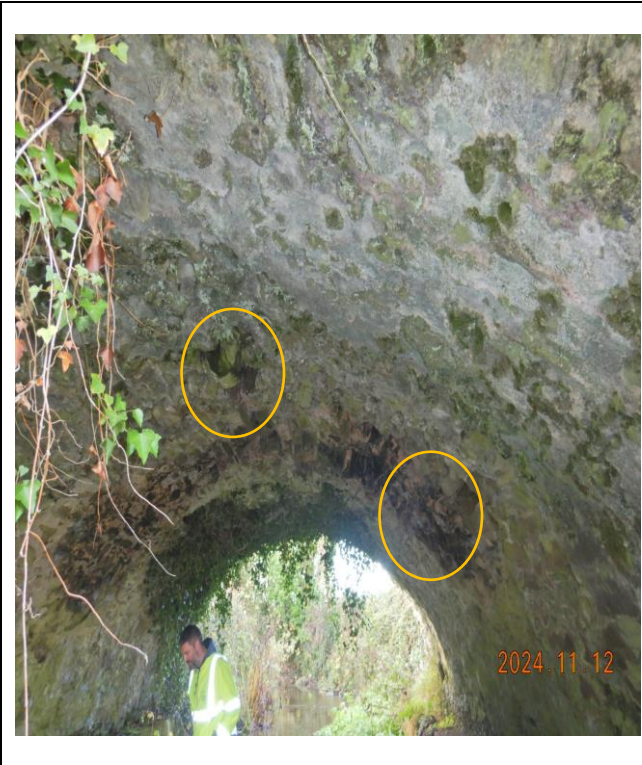
Areas of Dropped Stones to Arch Barrel
