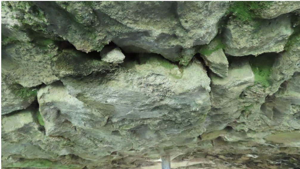
Photo 4 – crack in stonework of dry arch
