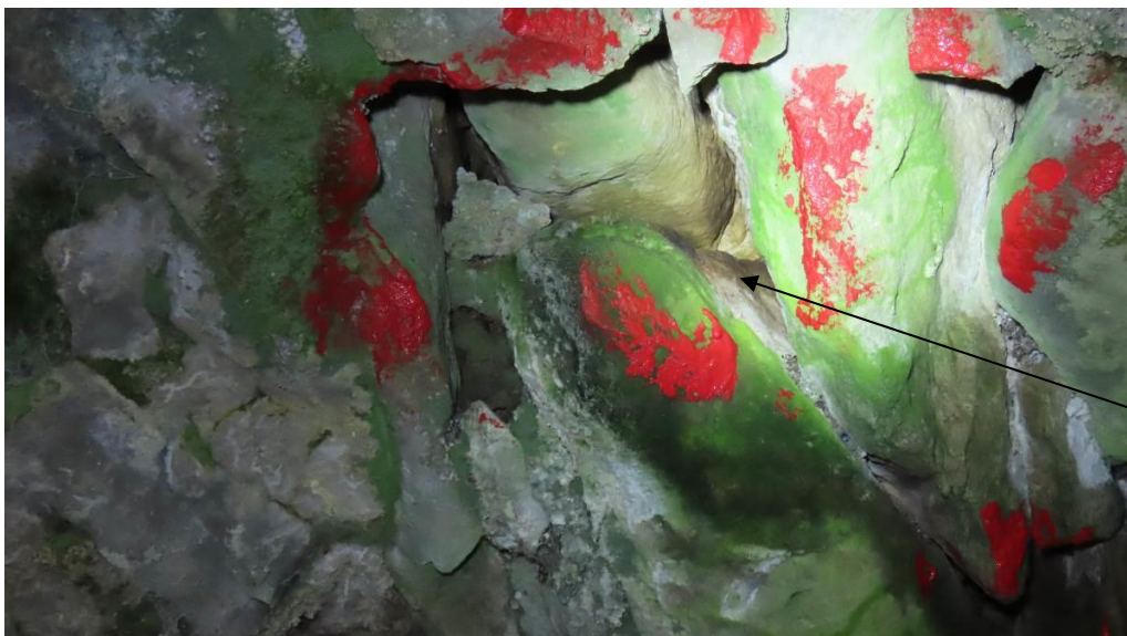
Photo 10 – staining from bats in crevice
