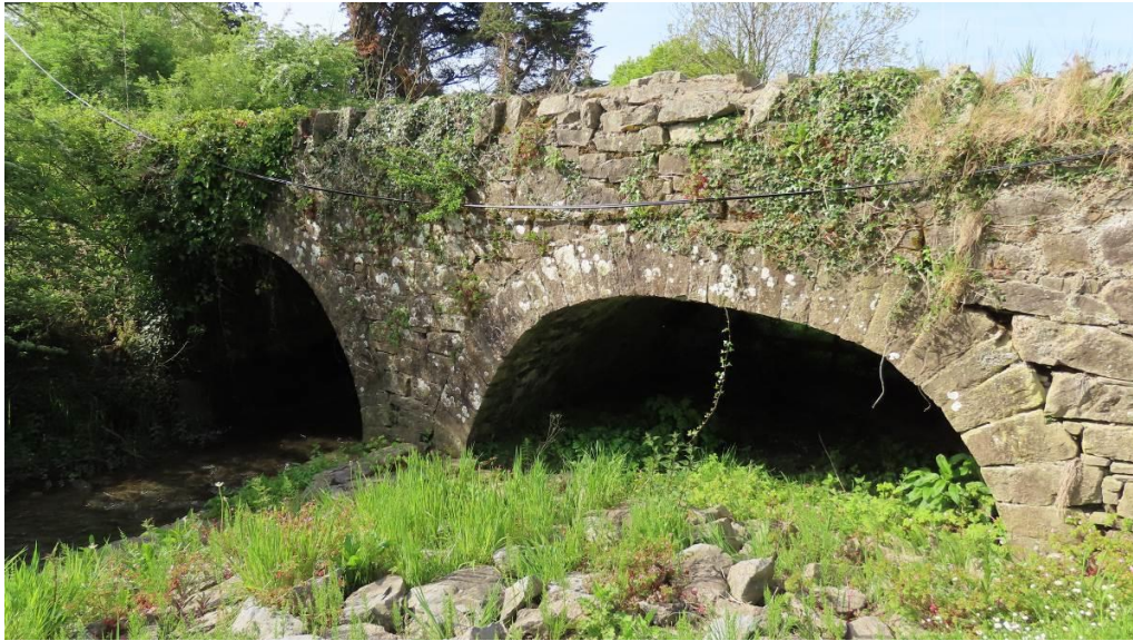
Photo 7 – upstream face of bridge showing damage to parapet wall
