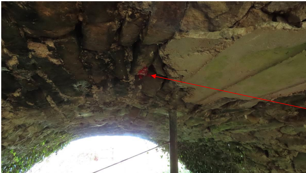
Photo 6 – crevice containing single bat under dry arch beside previous concrete repairs
