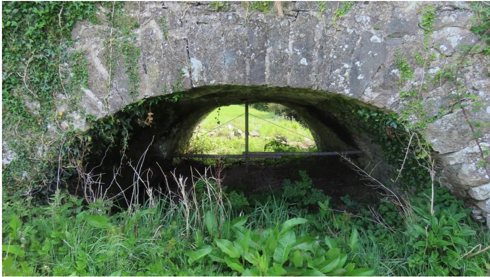
Photo 3 – dry arch 1m above level of watercourse. Metal prop under arch
