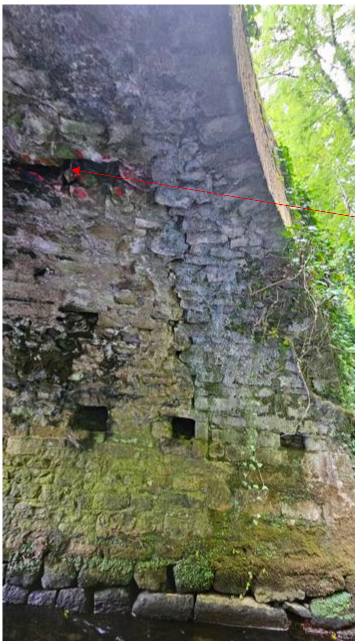
Photo 4 – view under southernmost arch showing circumferential crack running around the arch barrel and the position of the nursery colony of Daubenton's bats in a void under the arch
