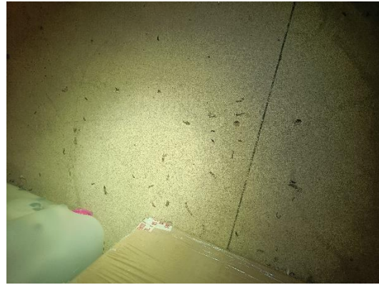
Plate 3-10 Small accumulation of droppings.
