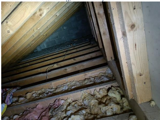
Plate 3-3 Dark sections present in the attic.
