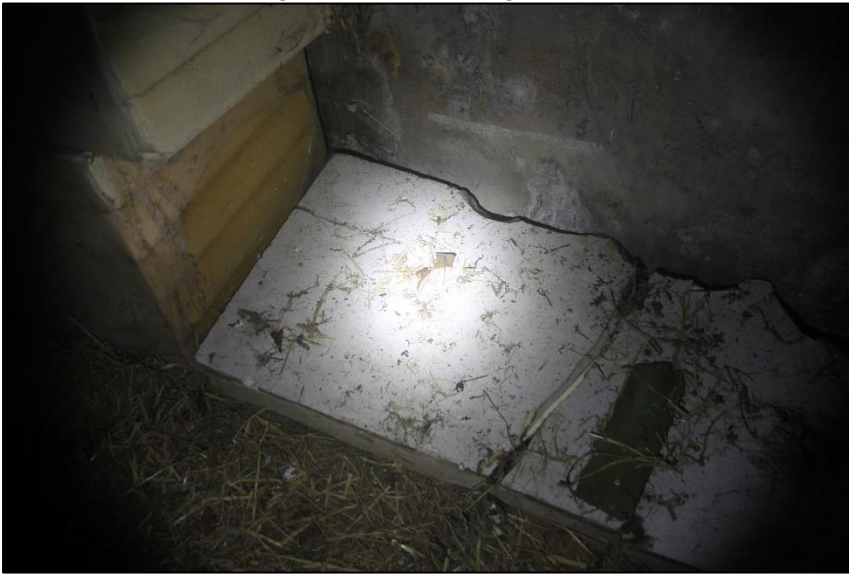
Plate 21 Building 1 Interior with bat droppings – August 2024
