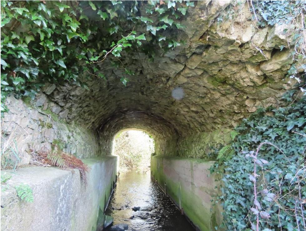
Photo 22 – view under arch from downstream elevation. High concrete plinth at the base of both abutments
