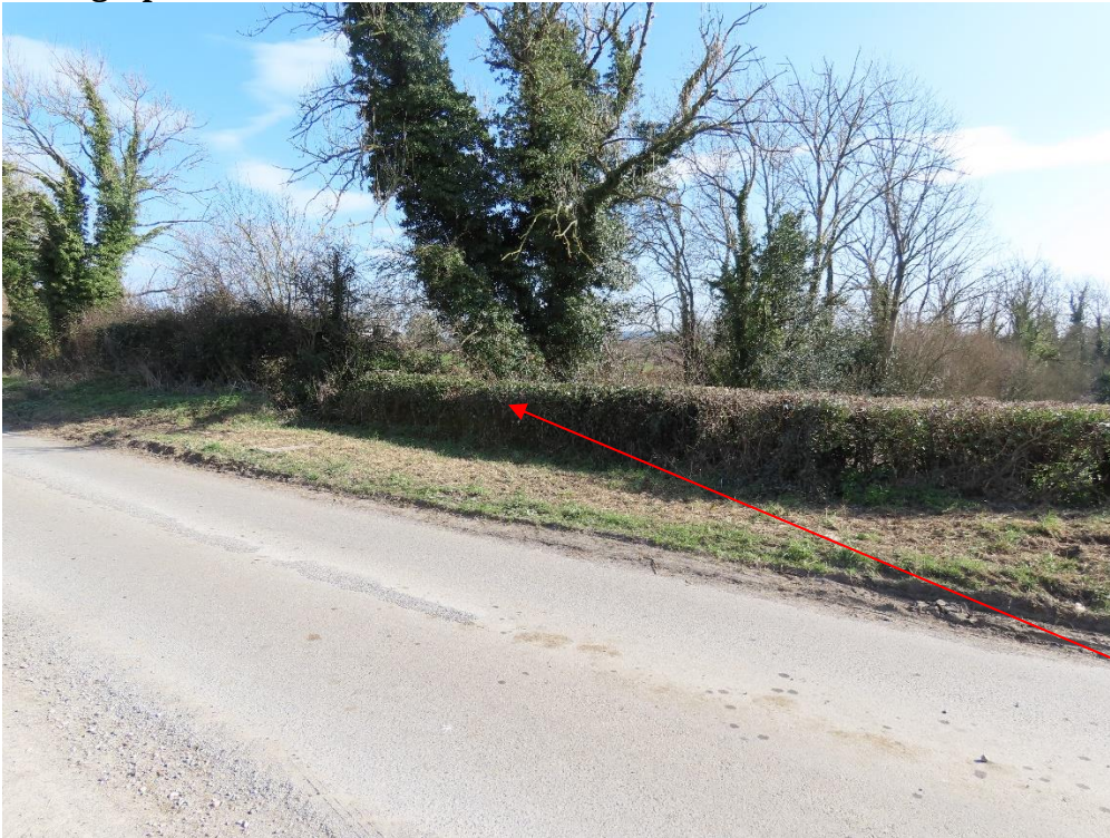
Photo 16 – downstream (southern parapet wall overgrown with vegetation
