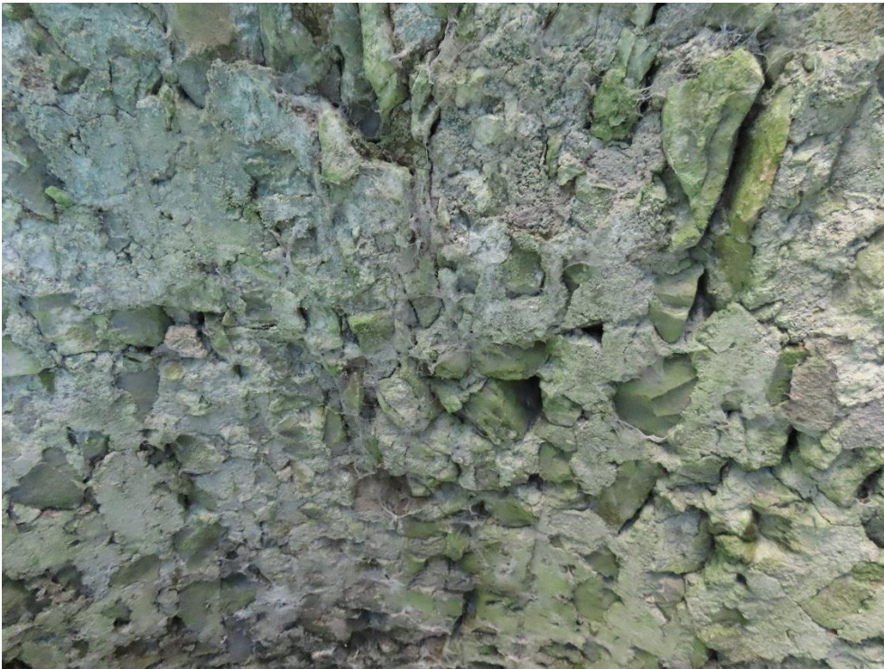
Photo 23 – previous repointing with cement under arch
