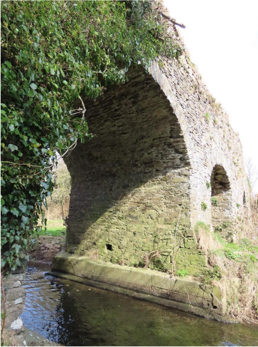
Photo 12 – ivy growth at downstream face of Arch 2
