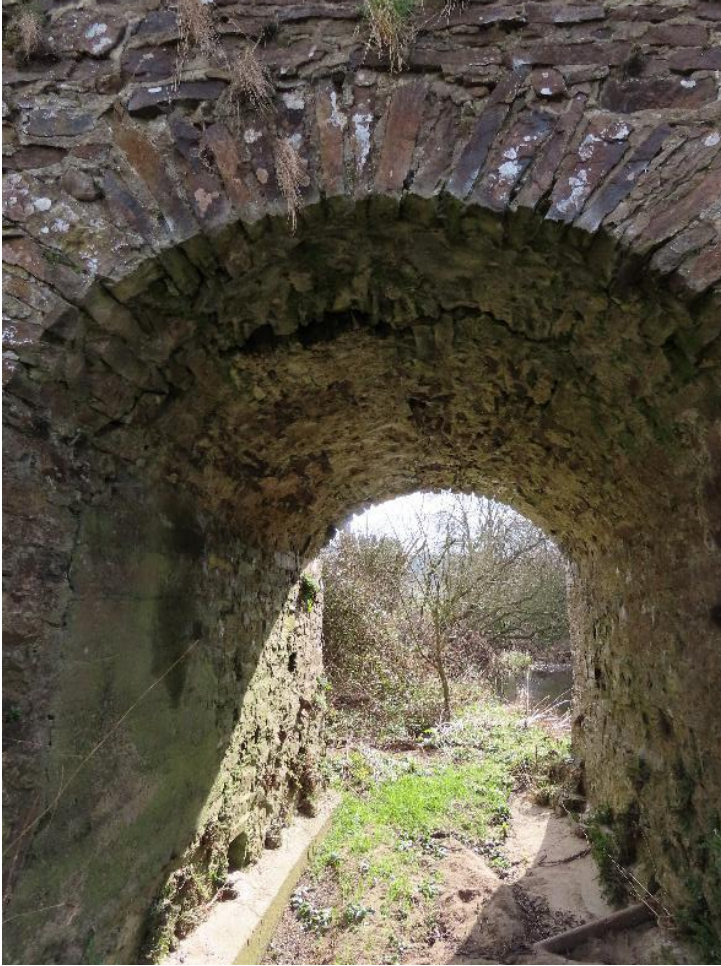
Photo 10 – view under Arch 3 showing large fissure running around arch barrel
