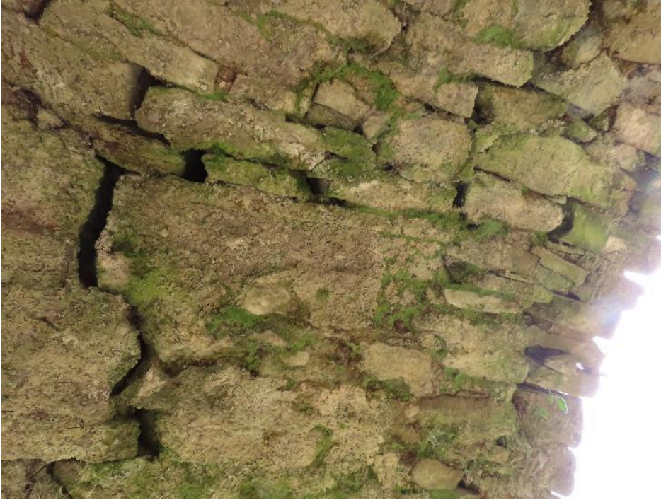
Photo 7 – fissure running under arch 4
