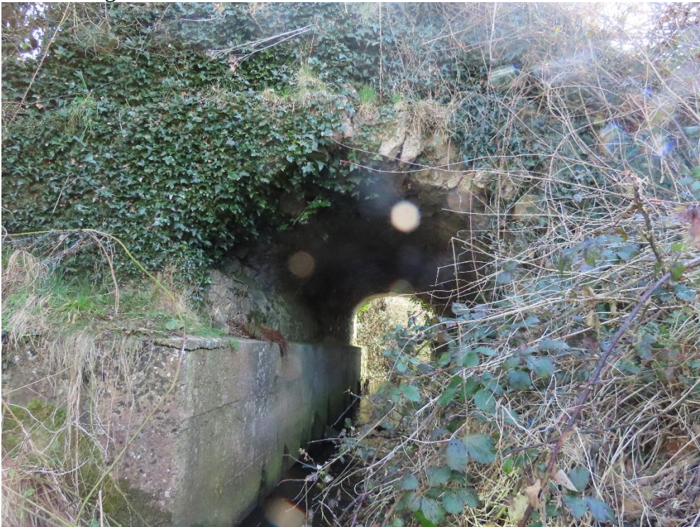
Photo 19 – downstream elevation of arch with damage to apex of arch
