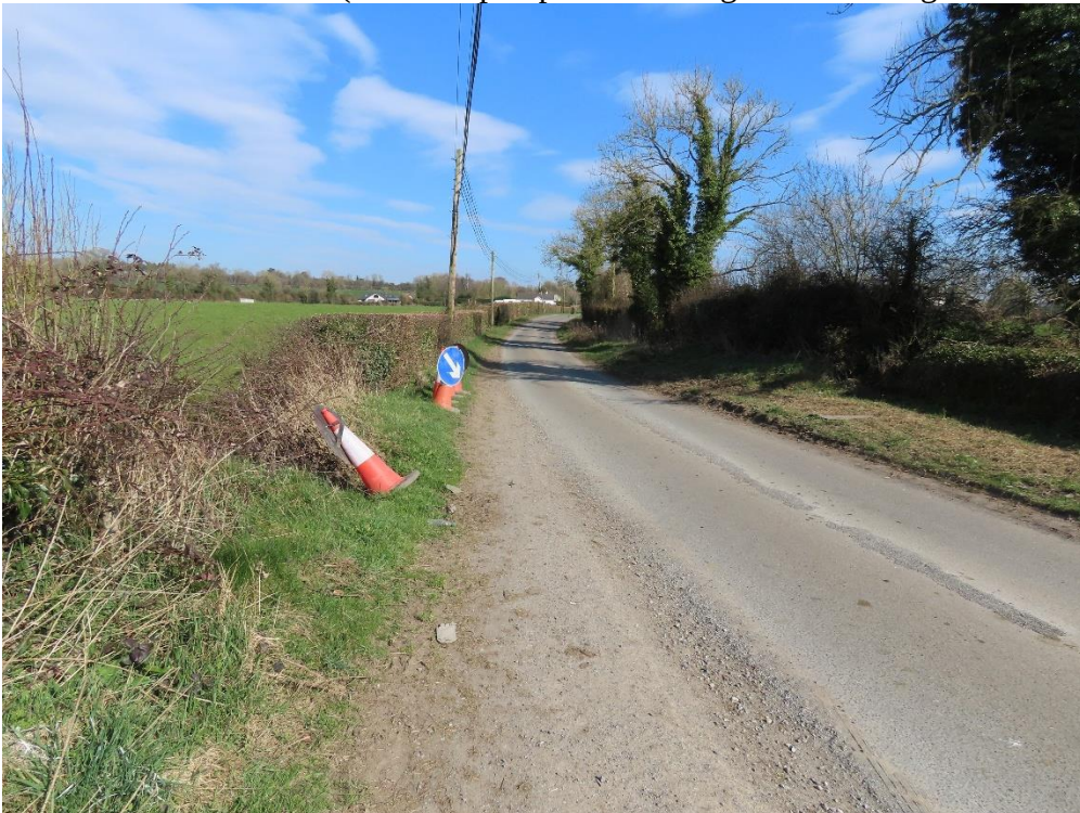
Photo 17 – bollards on upstream (northern) side of road to prevent traffic driving too close to damaged section
