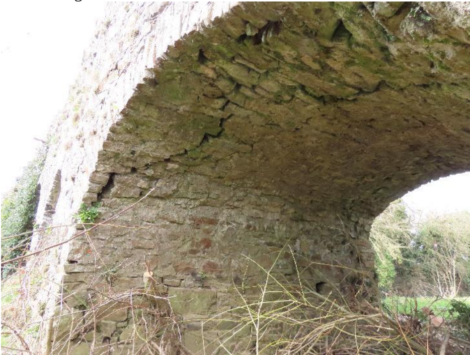
Photo 6 – crack running around arch barrel of Arch 4
