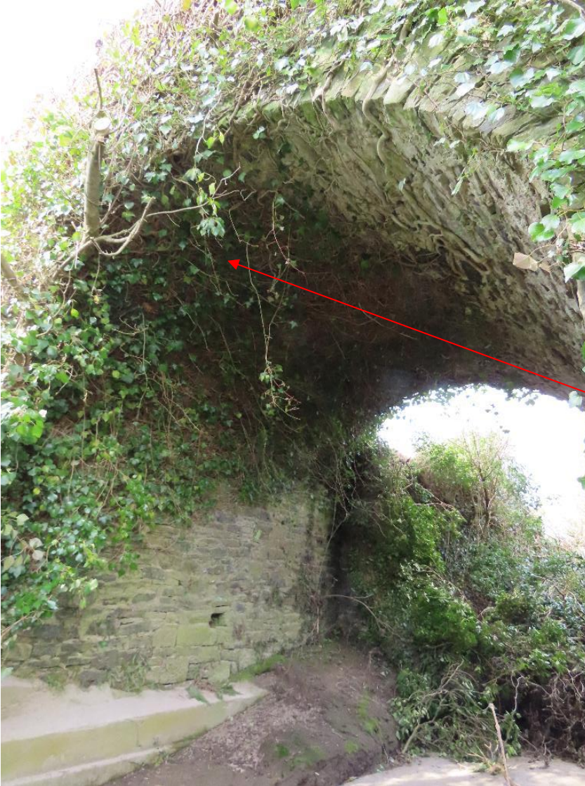
Photo 13 – heavy ivy growth under Arch 1. Old bird's nest in ivy
