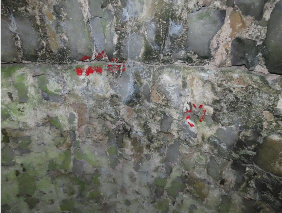
Photo 27 – section of expansion joint and another crevice marked for retention for bats
