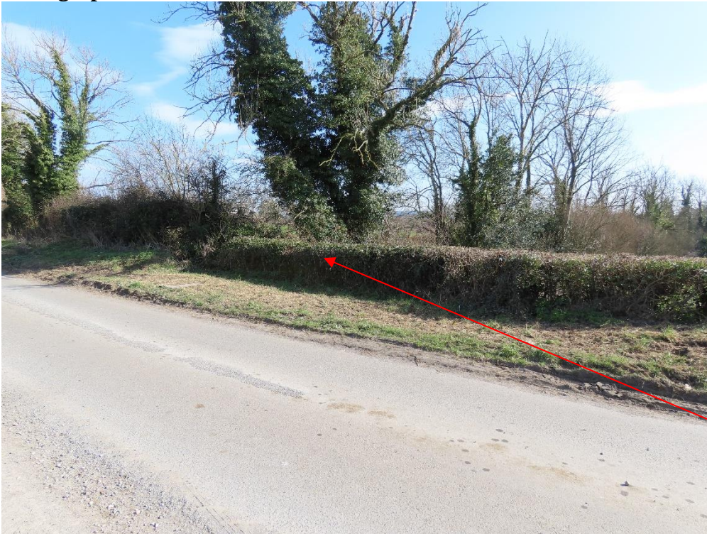
Photo 16 – downstream (southern parapet wall overgrown with vegetation
