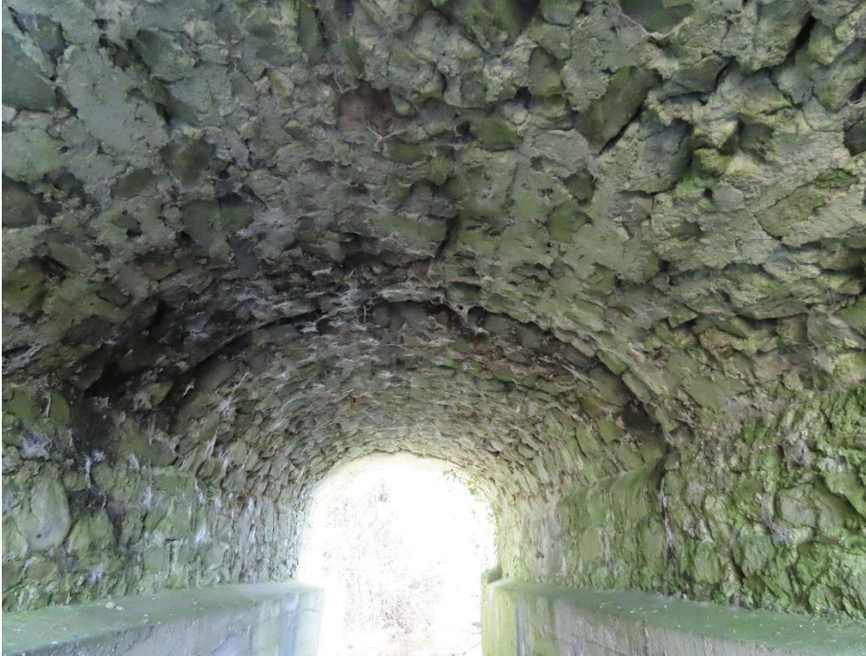
Photo 24 – extension joint midway under arch where bridge was effectively doubled in width in the past
