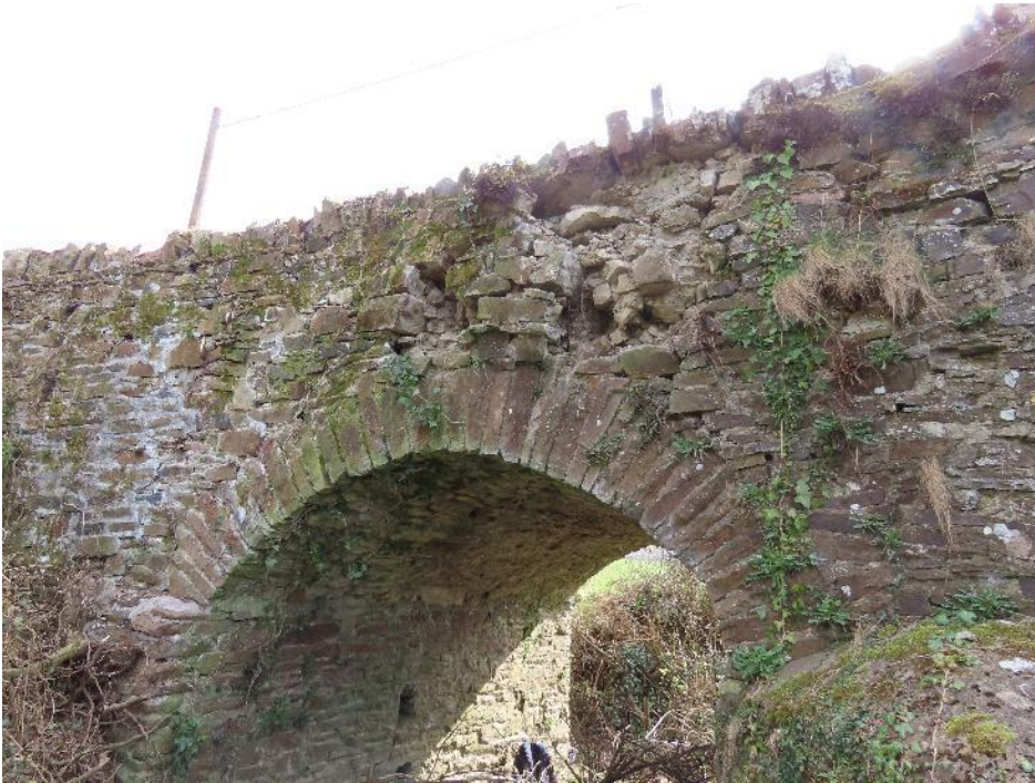
Photo 9 – damaged section of bridge parapet and spandrel wall above Arch 4 on upstream side
