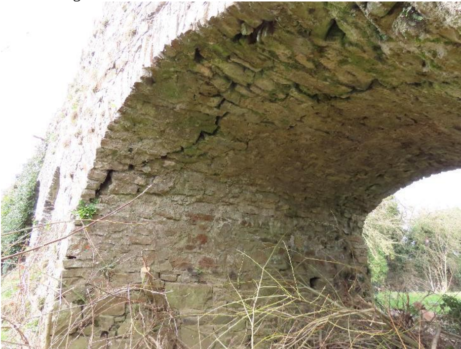
Photo 6 – crack running around arch barrel of Arch 4
