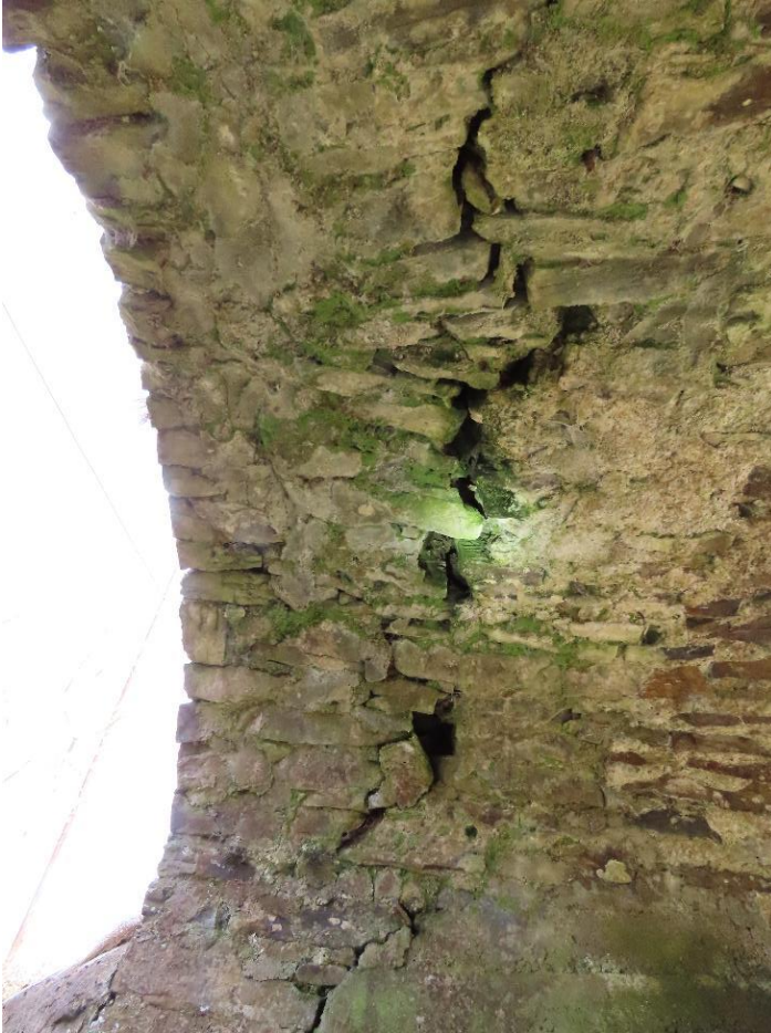
Photo 11 - close up of fissure under Arch 3
