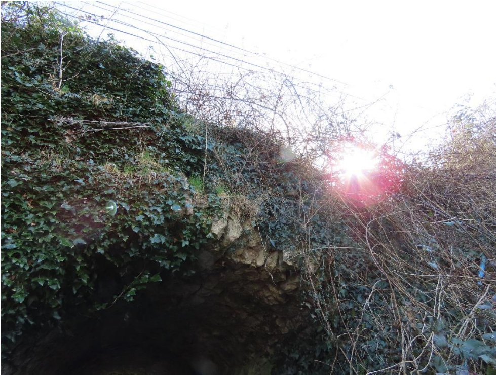
Photo 20 – close up of damage to stonework at apex of arch on downstream side
