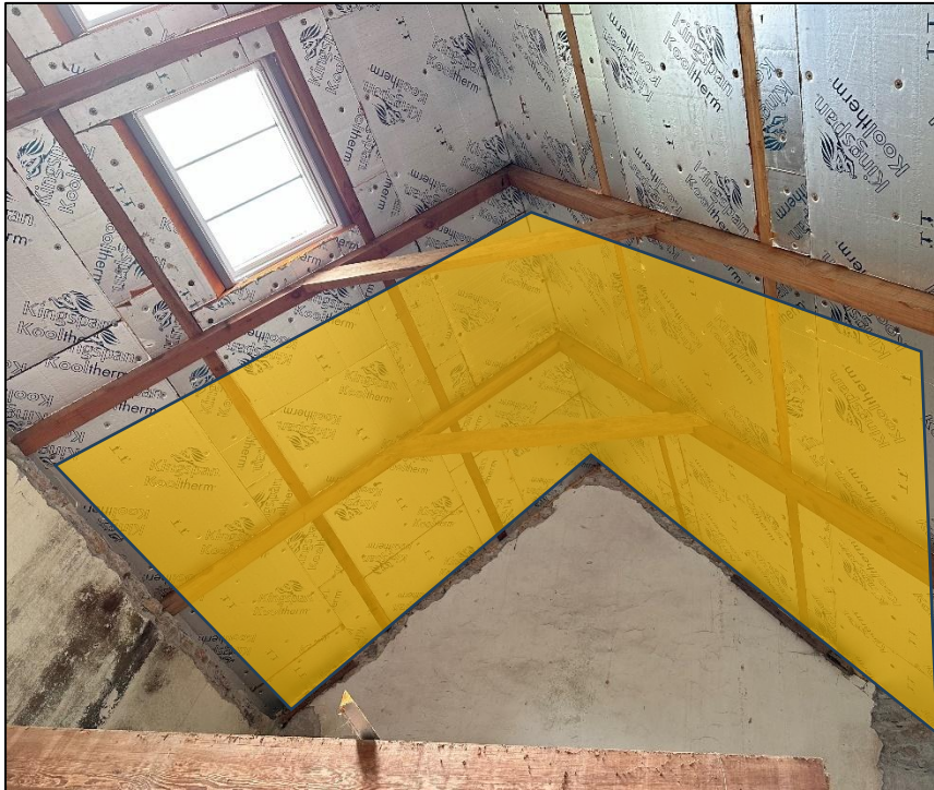
Figure 12: The primary bat colony has expanded into the space indicated in orange in 2024, with the colony occupying the same space occurring in an upstairs room on the opposite site of the gable wall
