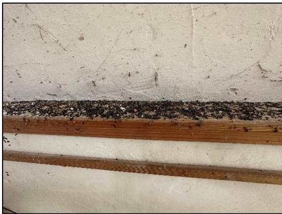
Figure 21: Evidence for a multi-species roost of bats was abundant throughout the barn block in the form of large amounts of droppings
