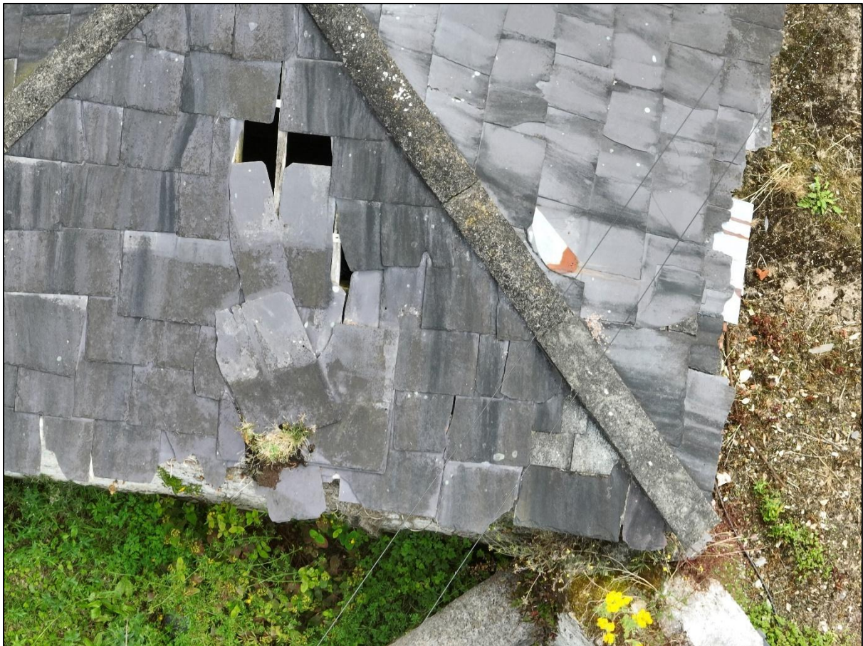
Figure 7: Aerial photograph of the roof of the milking parlour building, which urgently requires repair/re-roofing
