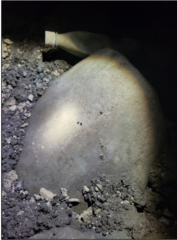
Plate 1 bat droppings found in ground floor of Lanistown Castle
