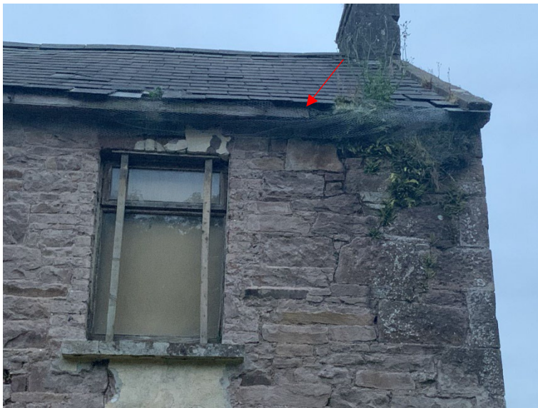
Plate 3-4: Gap under roof tiles
