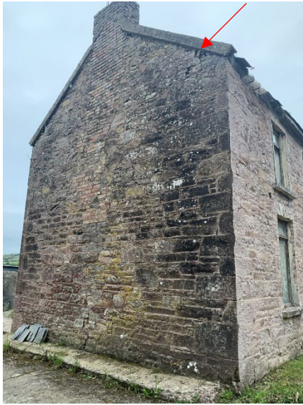
Plate 3-3: Gaps between stonework
