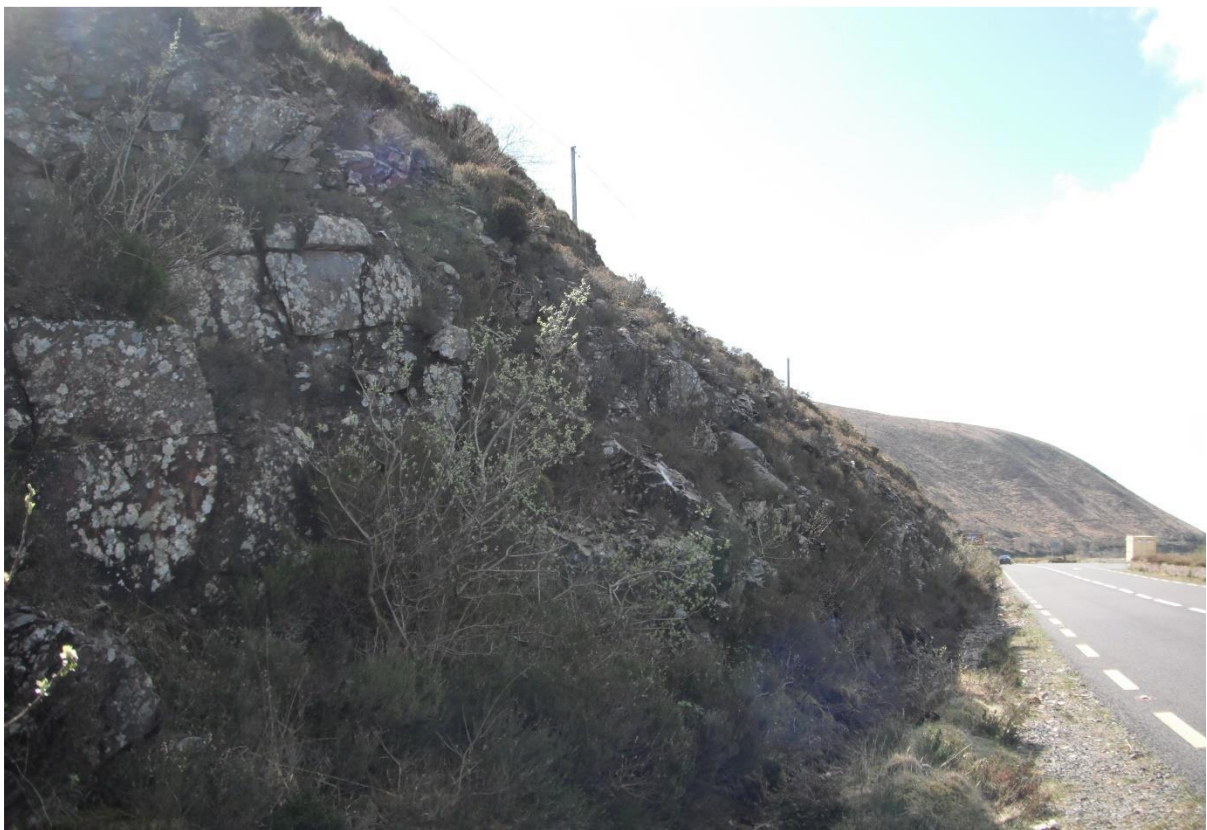
Plate 12: View west (towards Drung Hill Tunnels) showing existing profile with exposed rock and N70.
