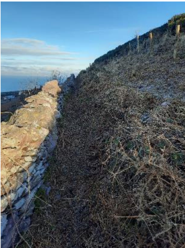
Plate 2. View from upper side of stone wall facing north
