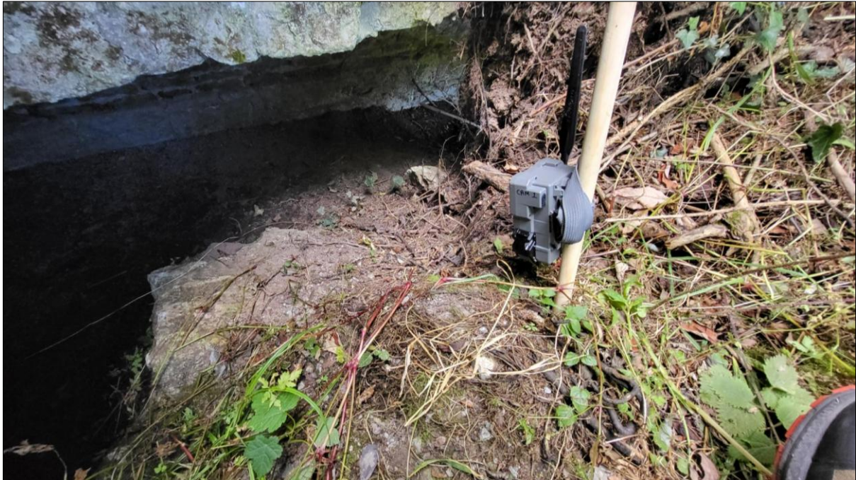
Plate 4.1 Otter couch (C2) located in a collapsed retaining wall near the railway, July 2026
