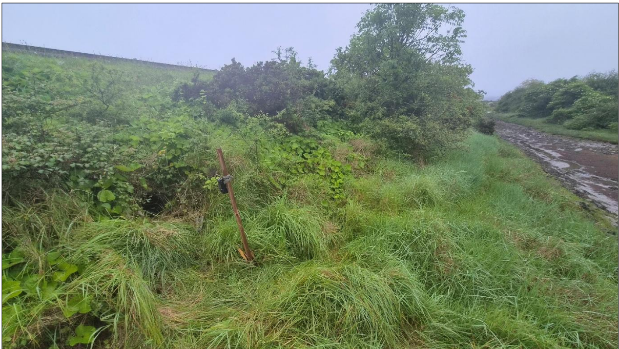
Plate 3.4 Mammal culvert connecting small lagoon to the Great Island Channel under the N25
