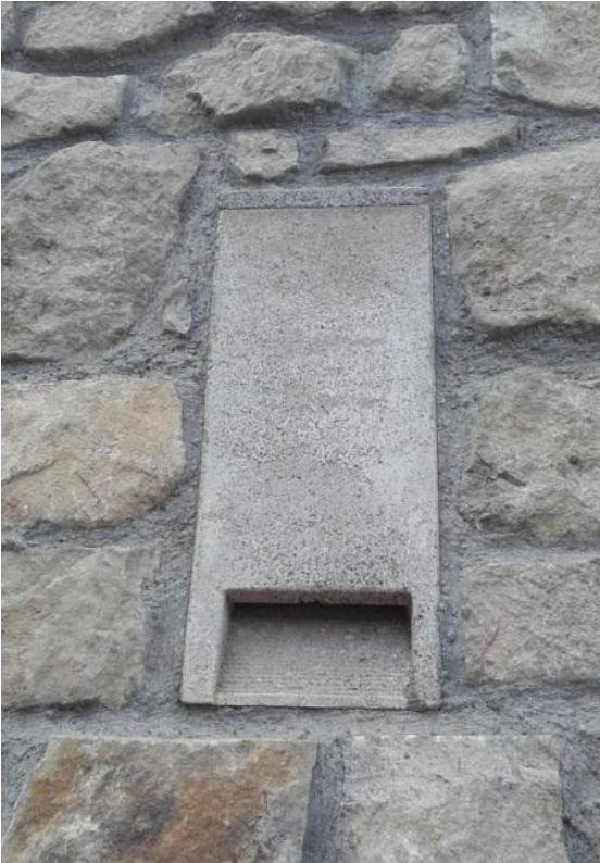
Ross Bridge, Co. Clare – bat tube built into the parapet walls of the bridge to provide replacement roosting for Daubenton's bats (Photo: Tina Aughney).
