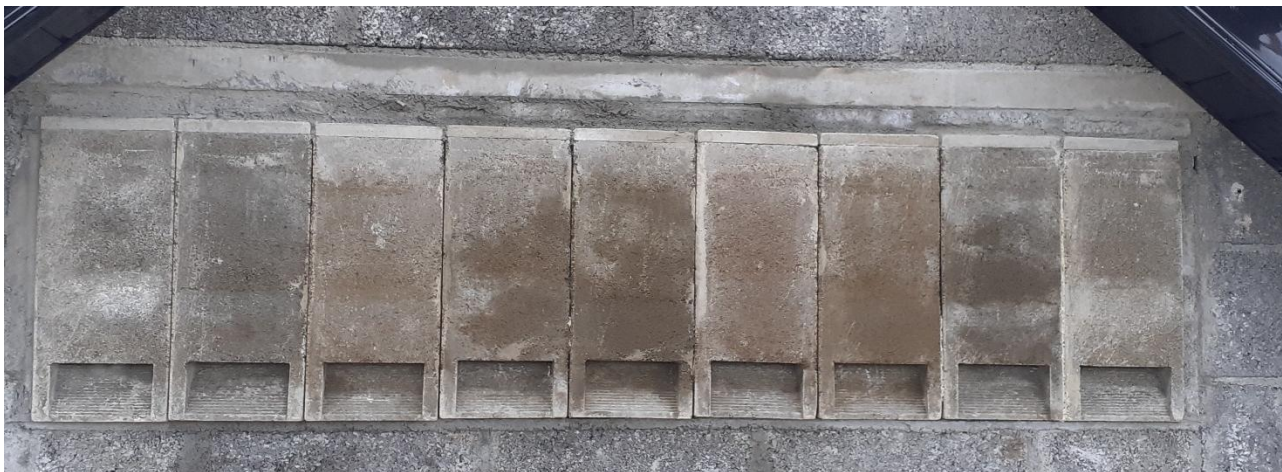
Series of Bat Tubes inserted into the external wall of Oldstreet Substation Bat House, Co. Galway (pre-plaster).
