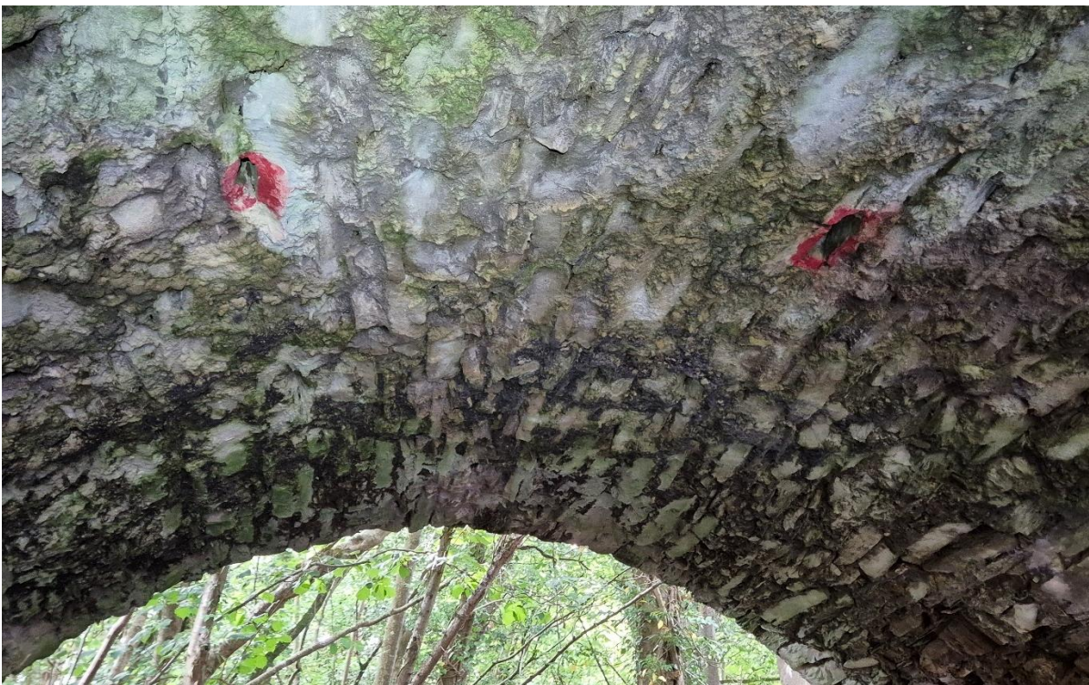
Plate 4-8: Bridge No. 8, Drumbeg, Co. Donegal – depicting the crevices, suitable for roosting bats, marked by red paint.
