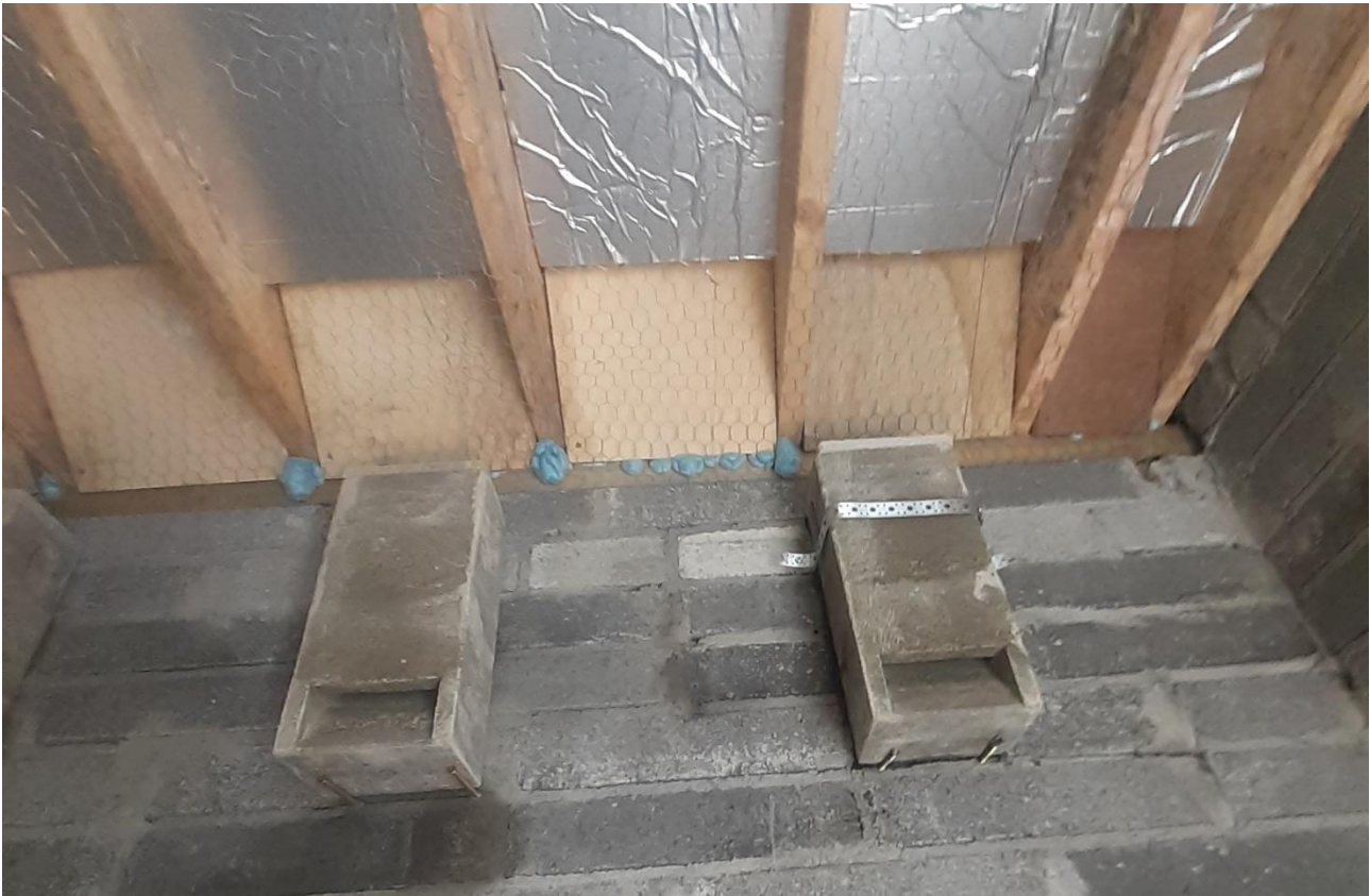
Bat Tubes fixed onto internal ground floor wall (Oldstreet Substation bat House, Co. Galway).
