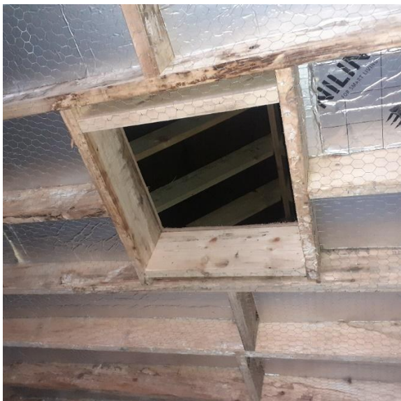
Internal open trap door and insulated ceiling (ground floor) of Oldstreet Substation Bat House, Co. Galway.
