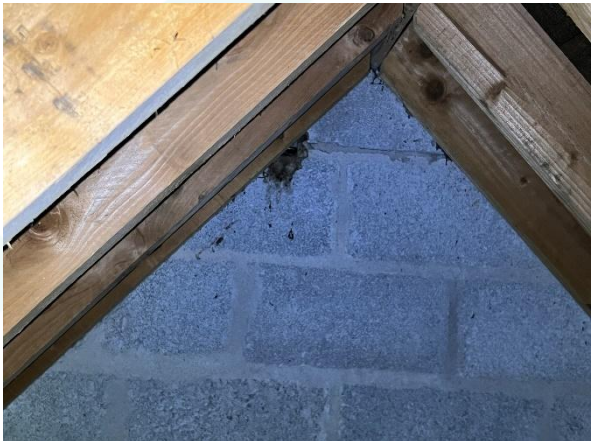
Plate 11 Hole in blockwork directly above accumulation of droppings
