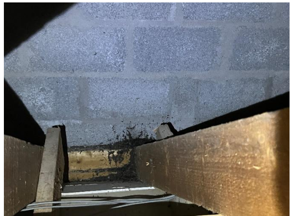
Plate 10 Large accumulations of droppings adjacent to carcasses along interior wall, west apse north elevation.
