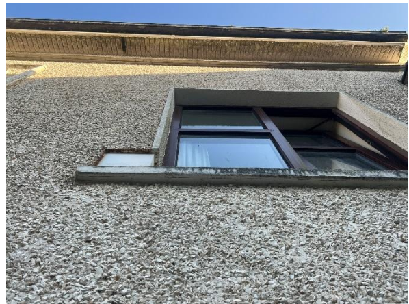
Plate 4 Bat droppings on windowpane adjacent to west apse soffit north elevation
