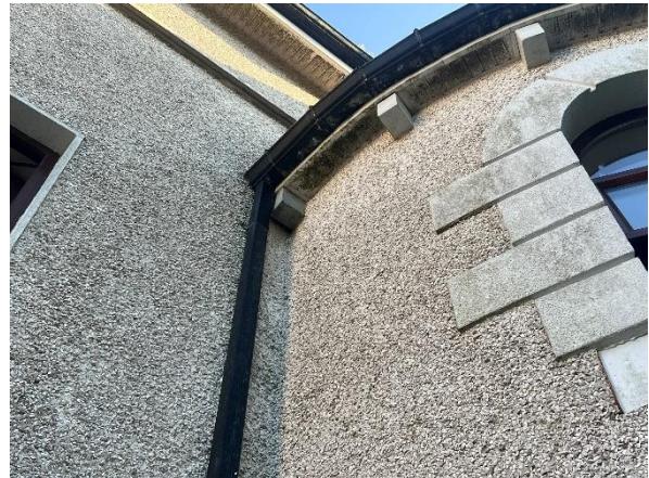
Plate 6 Vent-like Potential Roost Feature above droppings on west apse soffit.
