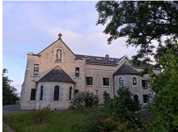
Plate 14 188 common pipistrelles emerging from vent-like feature (red) on west apse soffit.
