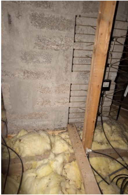
Plate 3. Pipistrelle droppings on insulation near chimney breast east side of building
