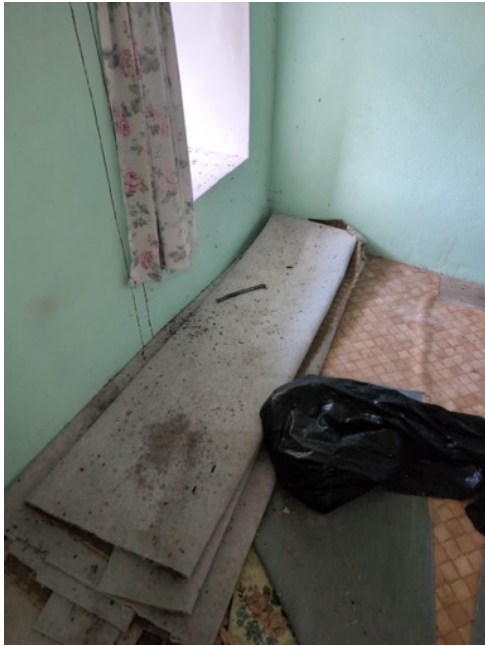
Plate 7. Bedroom to West extensive horseshoe droppings but relatively widely scattered. Extensive staining on western Gable probably indicative of location of Pipistrelle roost.
