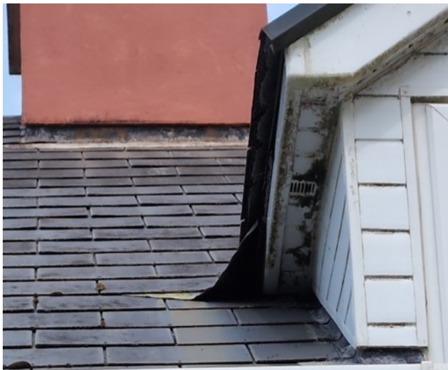
Plate 2. Front elevation of dormer windows facing south. Prominent flashing from which bats are emerging
