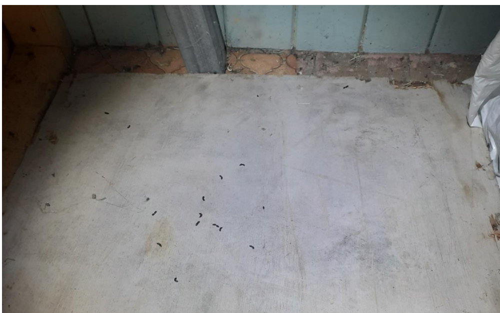
Plate 2: Lesser horseshoe bat droppings on floor of hot press in Building 1 (farm house - 21/7/22).
