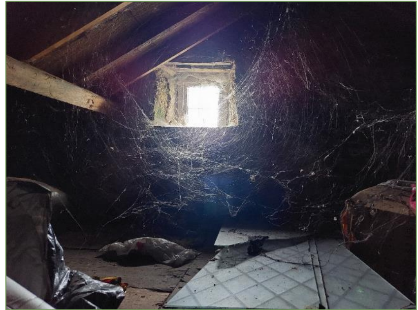
A14. View of the attic of the former residence showing heavily cobwebbed interior and light ingress.
