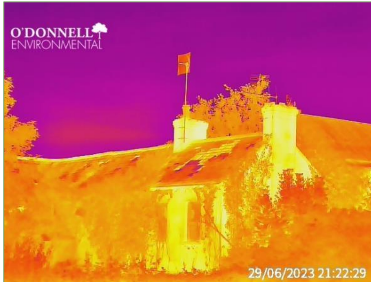
Plate 2.4 Example image from thermal camera covering the western aspect of Eastville House.
