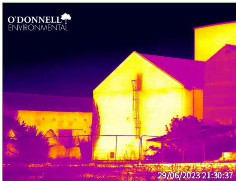
Plate 2.5 Example image from thermal camera covering the western aspect of the former mill buildings complex.
