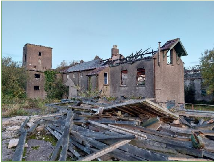
A1. View of southeastern portion of the mills complex showing extensive fire damage of the building.
