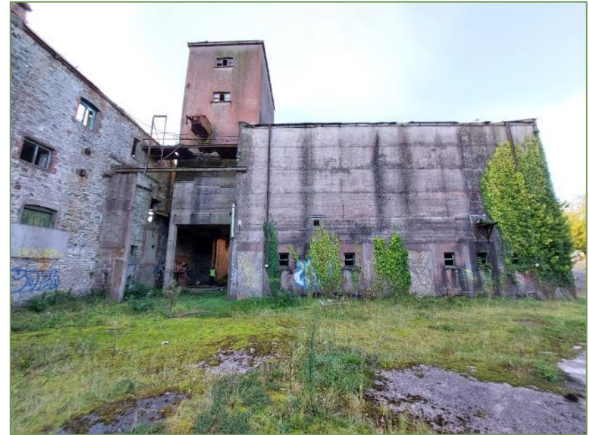
A4. View of the northern aspect of the concrete tower and associated concrete structures.
