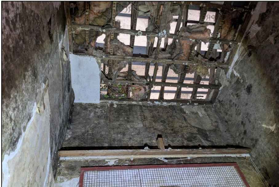
Plate 3-5. Interior roof space showing roofing membrane and water ingress.
