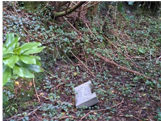
Plate 6 Fallen chimney capping at rear of courthouse.
