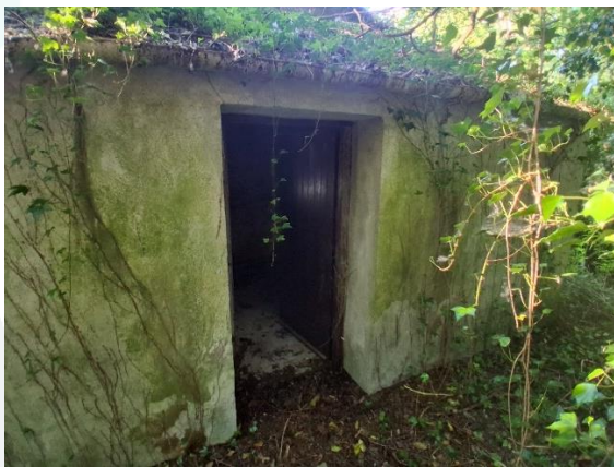
Plate 9 Open door at rear of structure providing access for bats.
