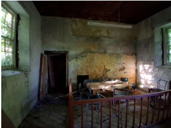
Plate 7 Interior of the courthouse showing miscellaneous debris to be removed as part of the proposed works.
