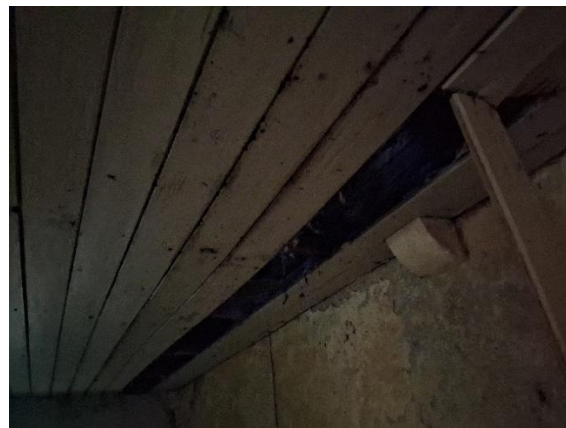
Plate 10 Broken ceiling panel allowing limited visual access into the attic space, as well as a potential access point for bats.
