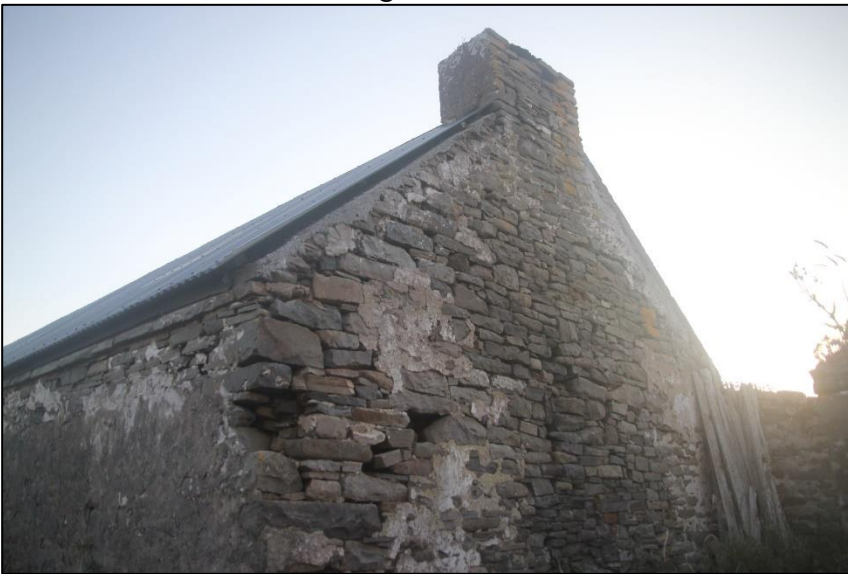
Plate 14 Gable of Barns for conversion. Cracks and crevices with bat roost potential.
