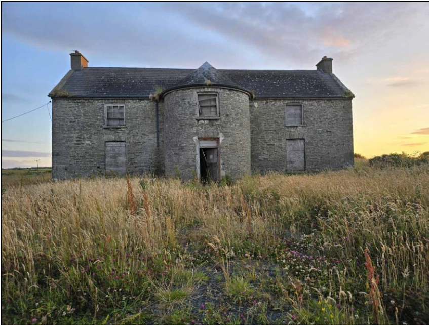
Plate 1 Front of Doonmore House onsite. Access available to bats via sides of tower giving it 'High' bat roost potential.
