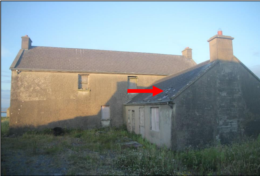
Plate 5 Rear of Dunmore house with old extension also shown. Access available via missing slates with emergence noted.
