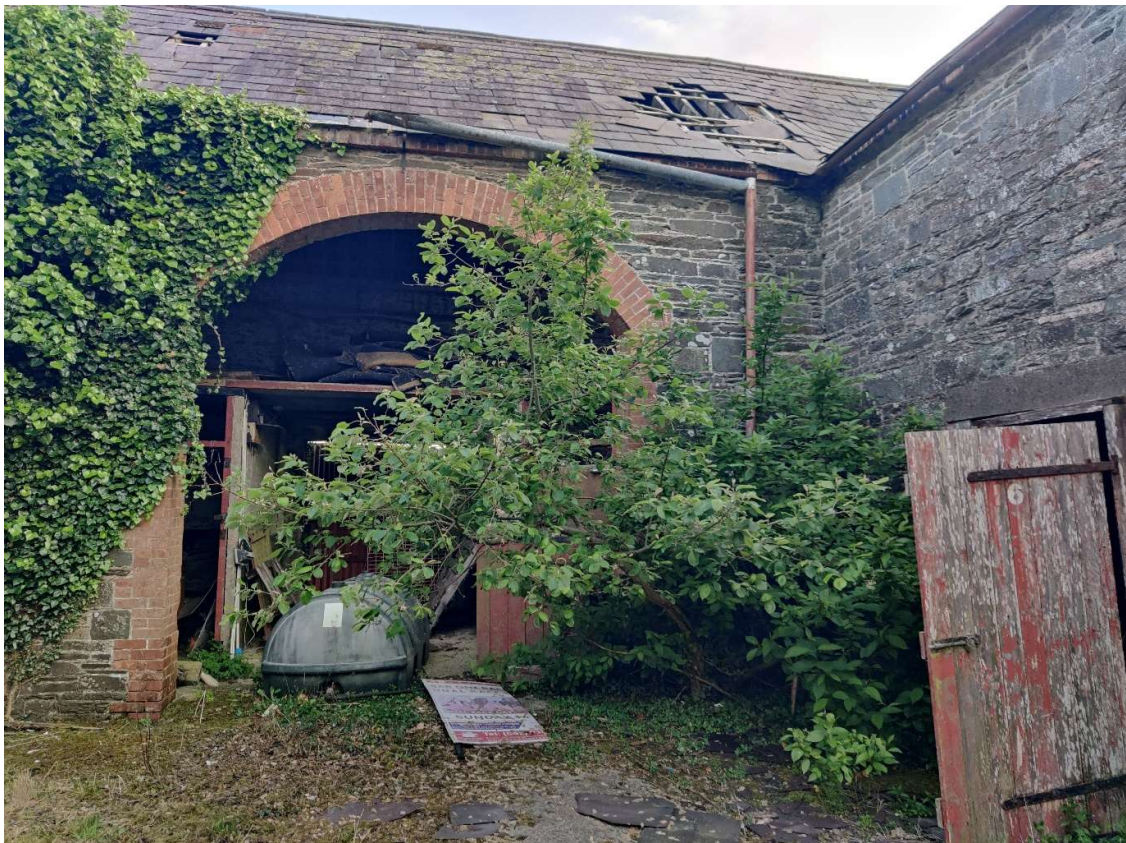
Plate 4. Gaps in slate roof tiles
