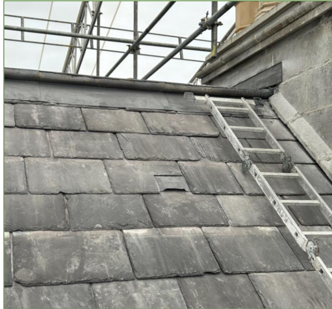
Plate 5.2 - Example of a lead bat access tile.
