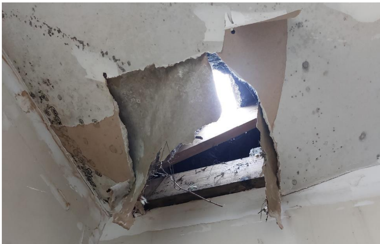
Plate 17: Fallen ceiling of office 7 (1)
