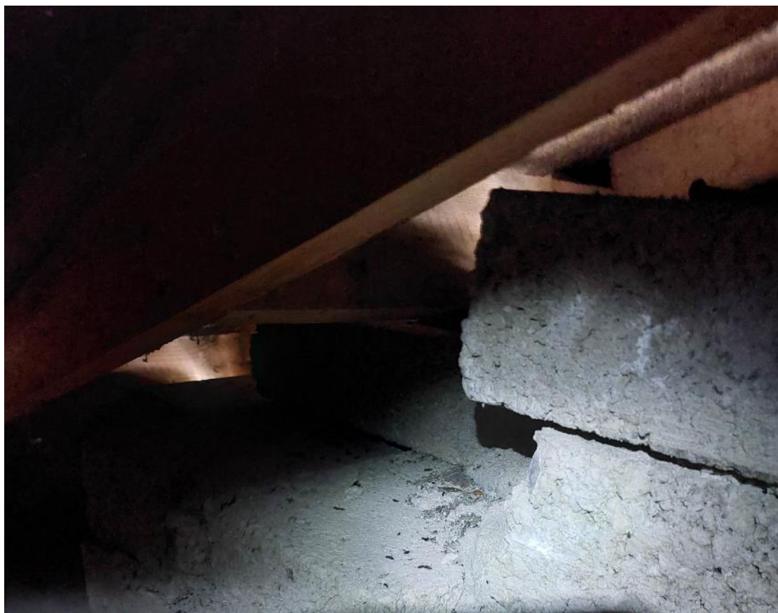
Plate 21: Fresh bat droppings on blocks which appear to connect to the external fascia
