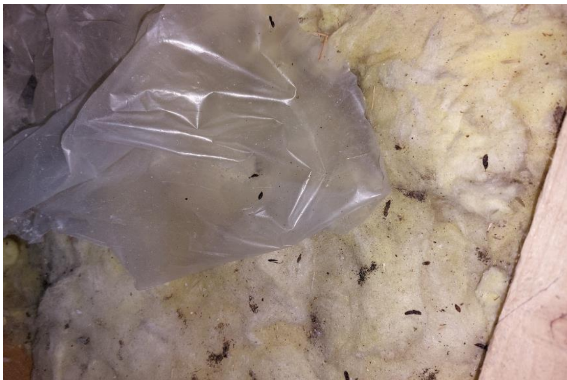
Plate 22: Bat droppings on insulating material in the building roof
