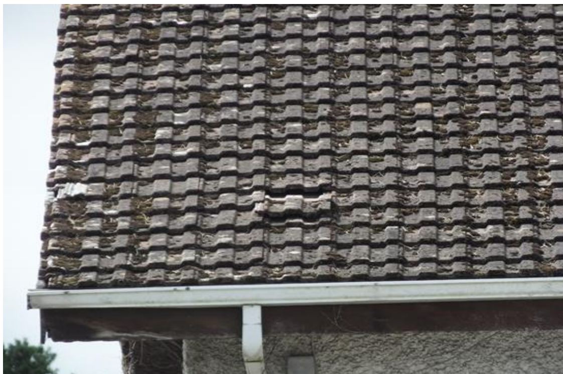
Plate 10: The damaged tiles at the south end of the building (1)
