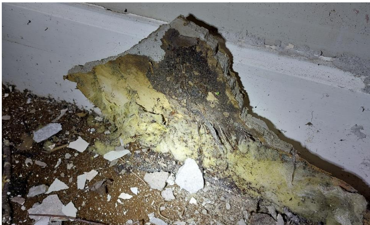
Plate 16: Fallen ceiling in office 7: Debris but no bat droppings present (1)
