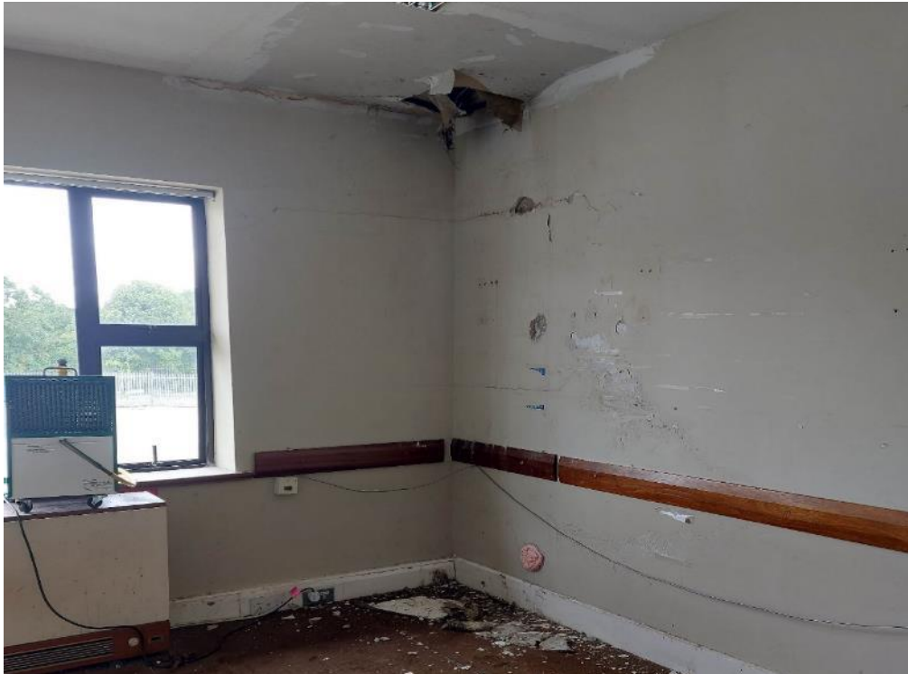
Plate 9: Damage in Office 7, 2 nd floor at South end of building (1)
