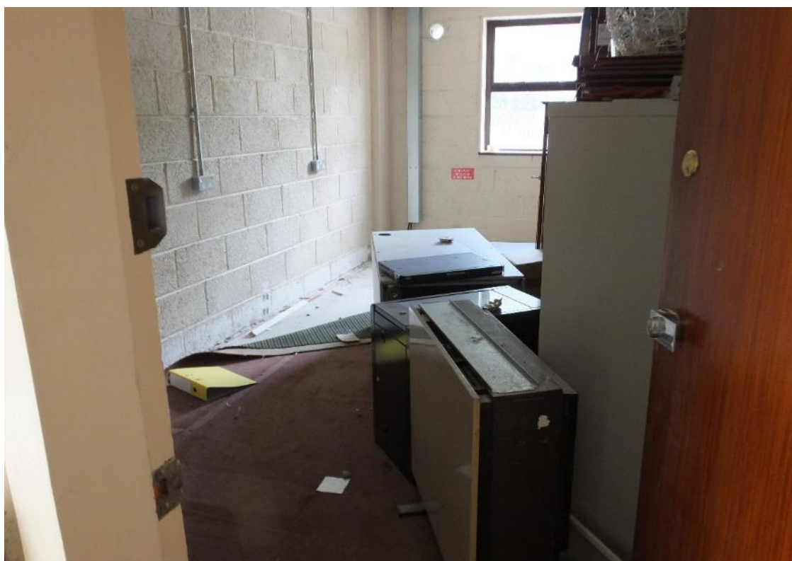
Plate 5: Office rooms with empty air vents (access outdoors)
