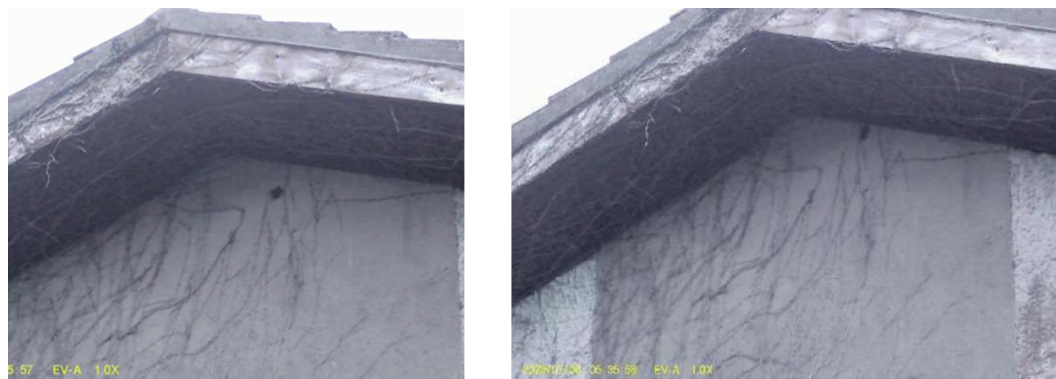
Plate 25: Soprano pipistrelle entering through gap in the roof eaves 5.35am, dawn survey
