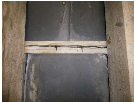
Photo R_4 Light slating battens and nails have split the batten
