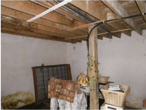
Photo F_1 Timber post/ wall stain to be reviewed
