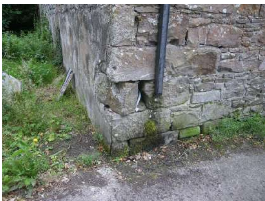
Photo E_8 South East corner, corner stone knocked out to be reset stone
