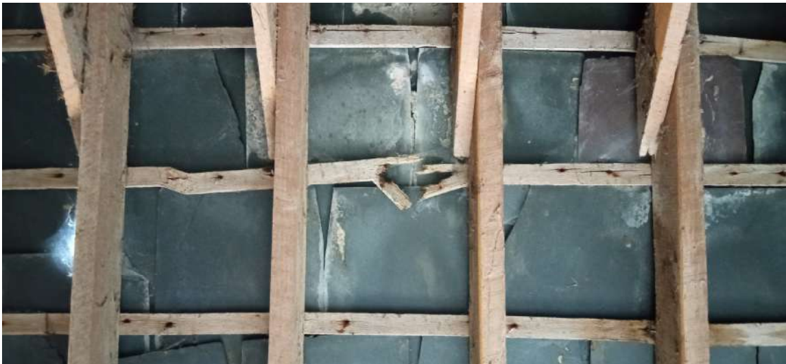
Photo R_5 Roof detail at collar – broken battens etc/ No sign of parging or torching having ever been done
