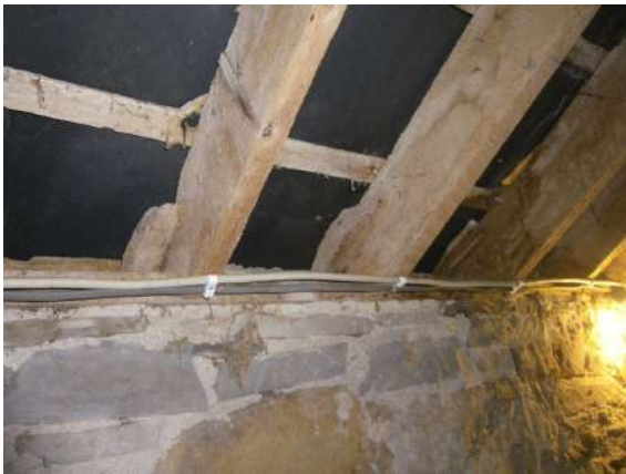
Photo R_3 Electrical cabling fixed along wallplate
