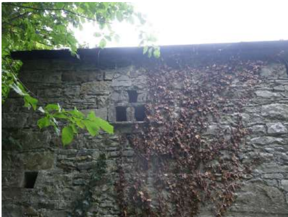
Photo E_4 South - Rear vent holes/ blocked up window
