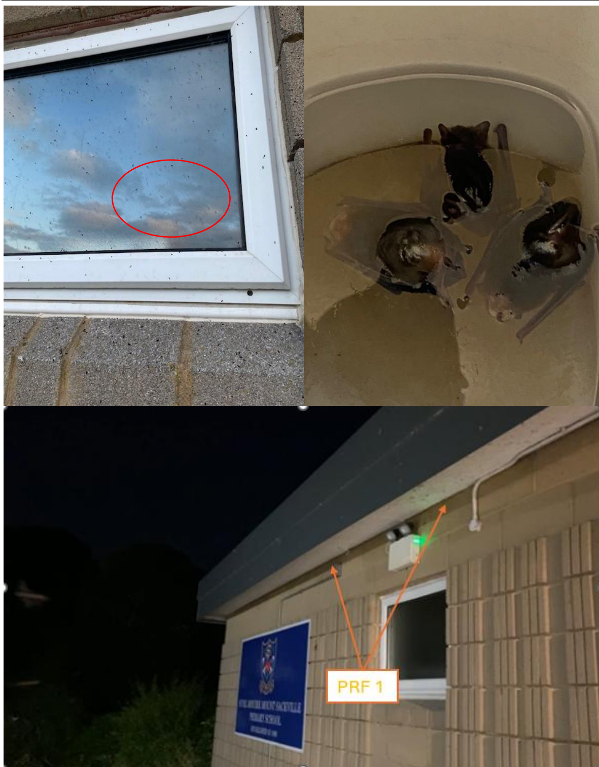
Plates 3&4&5 – Bat evidence in the form of droppings flecked onto window below roost entry point on northern side of building (top left) dead bats found in the bathroom on the northern side of the flat roof building (top right). Bat entry point (PRF1) above windows as shown between cavity block wall and flat roof (bottom)
