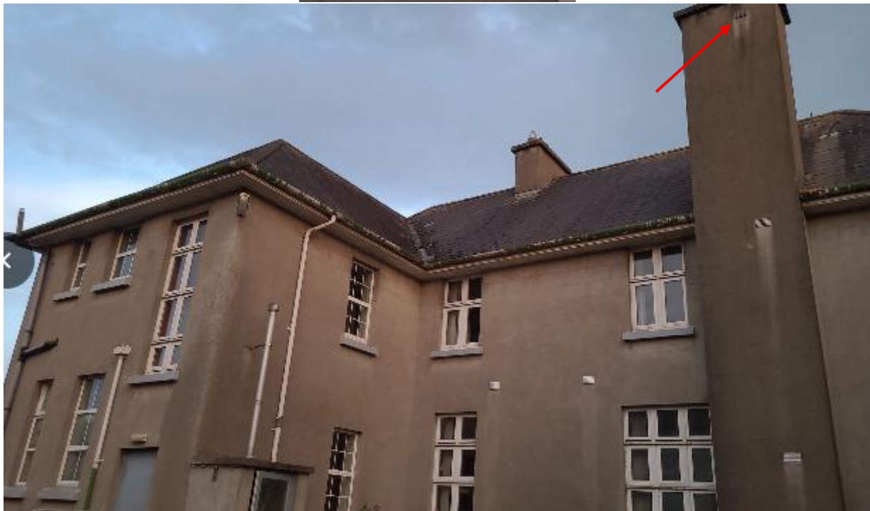
Bat roost entrance – See staining below roost entrance.
