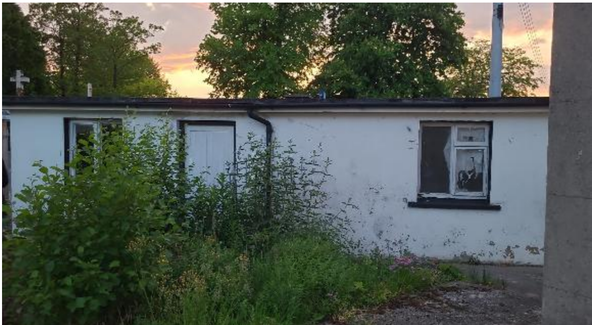
Garage – Flat roof, moderate bat roost potential.
