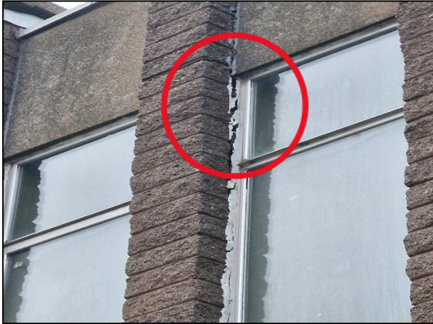
Figure 5: Active roost present on the western wall of the derelict garda station. Bats were observed emerging from the gap between the window frame and brick wall. This area is highlighted by the red circle. Photo taken on the 29 th of September 2025
