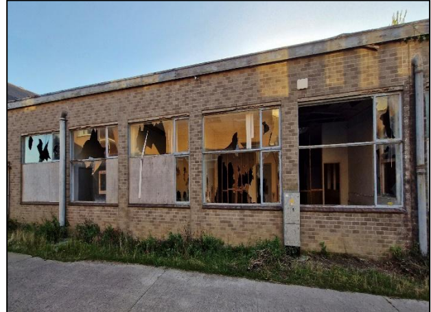
Figure 6: Potential roost features (broken windows) on single storey brick building. No emergences from this building were recorded during the 2025 survey period. However, one emergence was recorded in the 2022 survey. Photo taken on the 22 nd of September 2025
