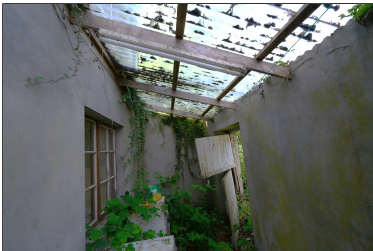
Plate 4 Outbuilding / extension area on the north side of the house (bat droppings found).
