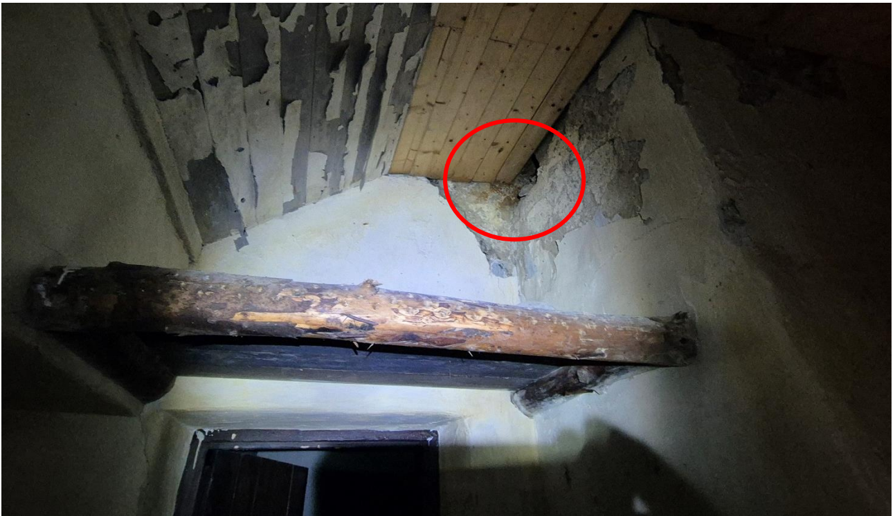
Plate 3d: Other potential bat access points to the attic of Gamekeeper's Lodge, Co. Wicklow with gap highlighted (room with fireplace).
