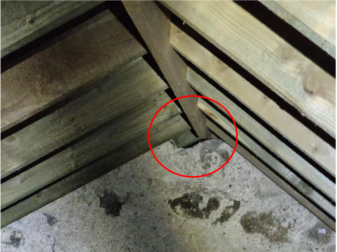
Plate 3c: Accessible attic of Gamekeeper's Lodge, Co. Wicklow with internal wall and gap highlighted.
