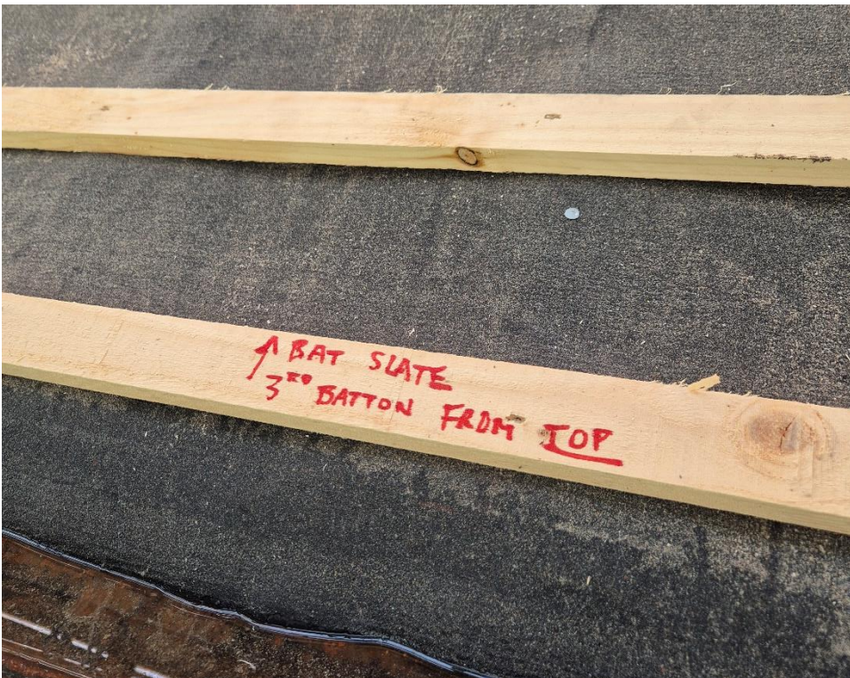
Bat specialist marked up where bat slates (x5) are to be positioned in consultation with NPWS – Coole Park Visitor Centre, Gort Co. Galway.
