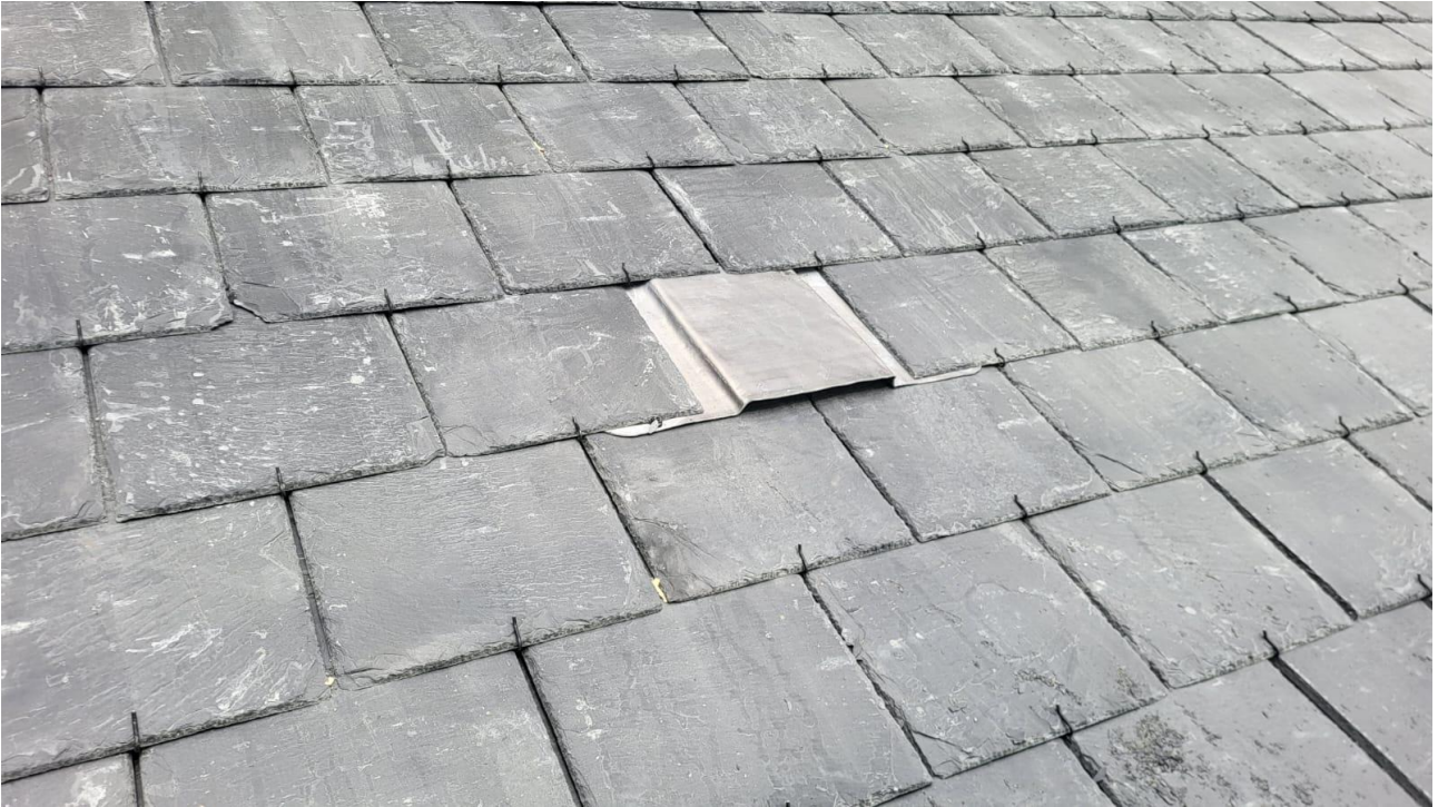
Bat slate in new roof (29.4.2025) of Coole Park Visitor Centre, Gort, Co Galway.
