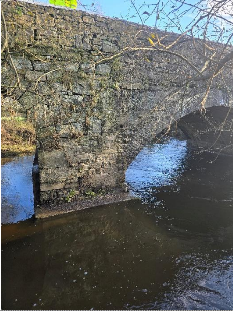
Photo 9 – Mortar loss from downstream spandrel wall.
