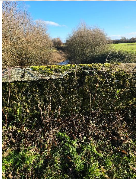
Photo 8 – Cracks and mortar loss from upstream parapet wall.
