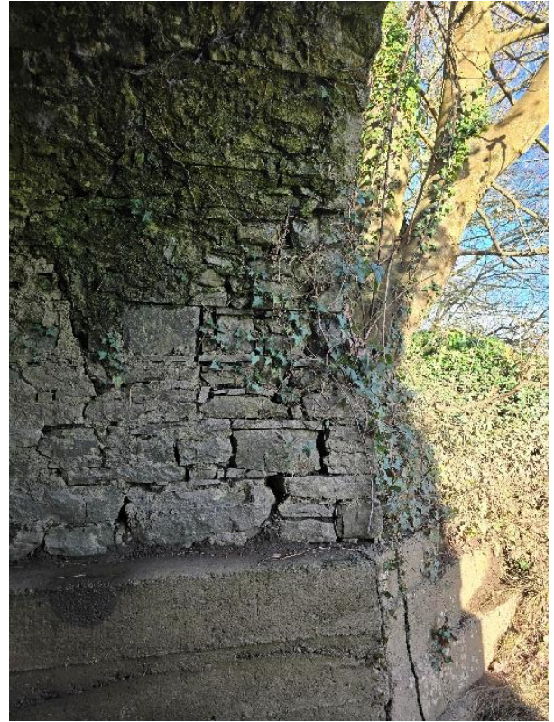
Photo 6 – Mortar loss from right-hand bank side of third arch.
