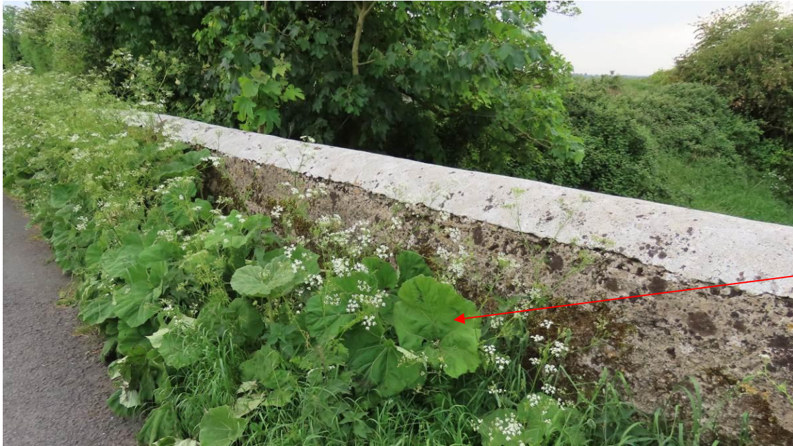
Photo 1 – winter heliotrope growing at base of parapet wall
