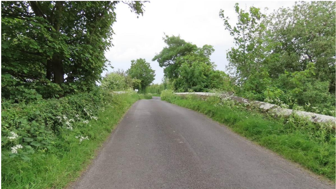
Photo 4 – parapet walls with vegetation growing at the base of both walls
