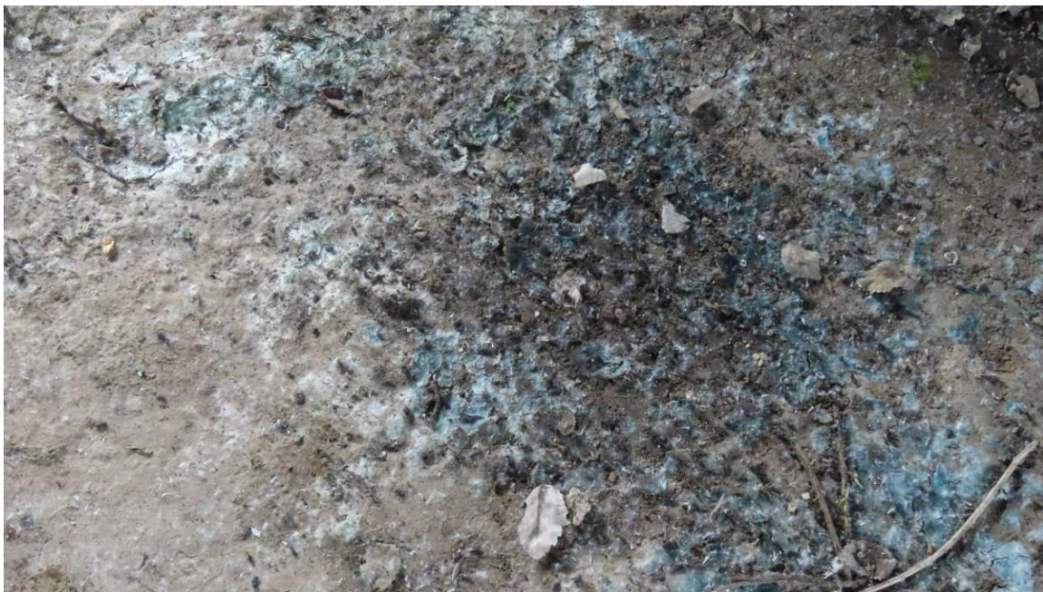
Photo 10 – large accumulation of bat droppings on cement floor of southernmost arch beneath construction joint
