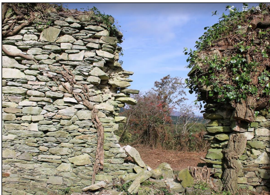
Plate 13: Collapsed window opening in N wall of church.
