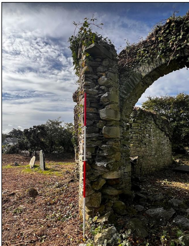
Plate 9: Southern wall of apsidal chamber which window has collapsed, facing southwest.
