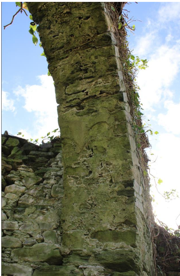
Plate 5: Mortar underneath chancel arch with possible plank centering visible.
