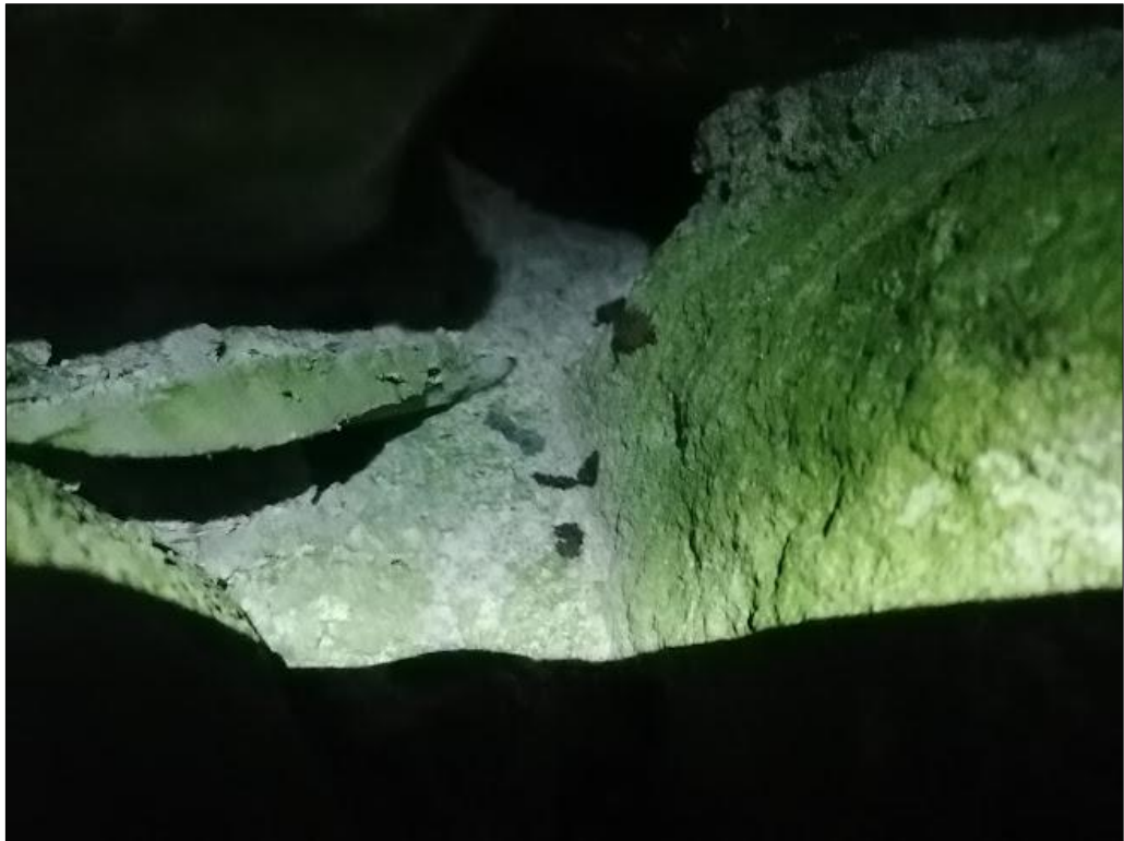
Plate 14. Bat droppings within the stone wall.
