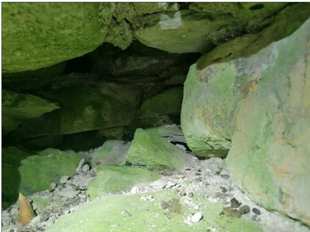
Plate 15. Bat droppings were noted within the stone wall along with mouse droppings.
