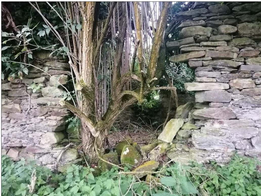
Plate 10. Elder bush growing in the collapsed church wall.
