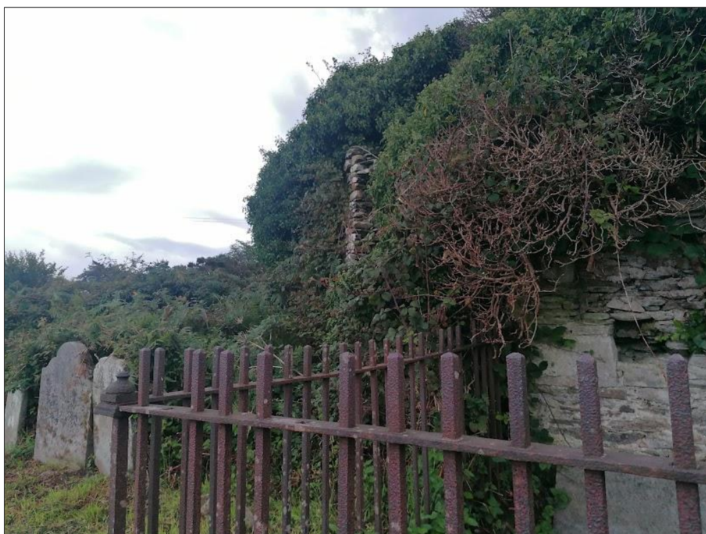
Plate 13. Extent of ivy on church walls obvious.
