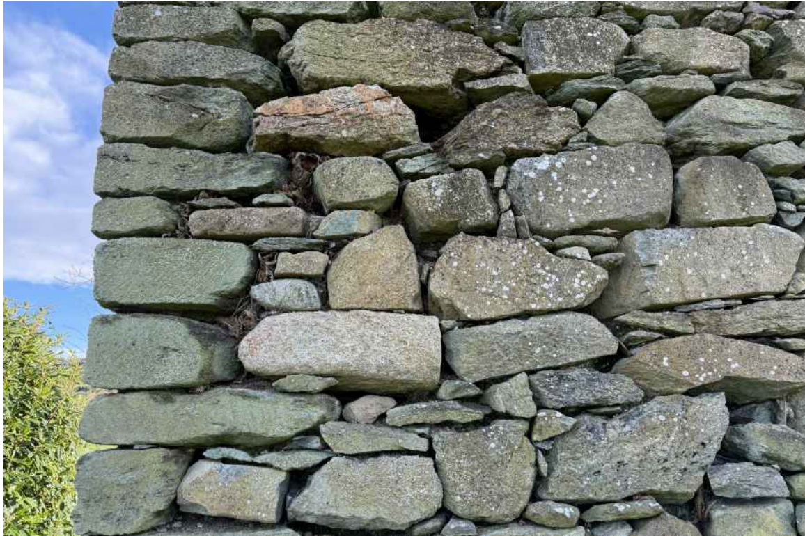
PHOTOGRAPH 3 - DEAD EMBEDDED IVY STEMS AND MISSING PINNING STONES
