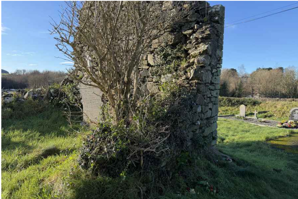
PHOTOGRAPH 9 - SAPLING GROWING FROM THE NORTH WALL
