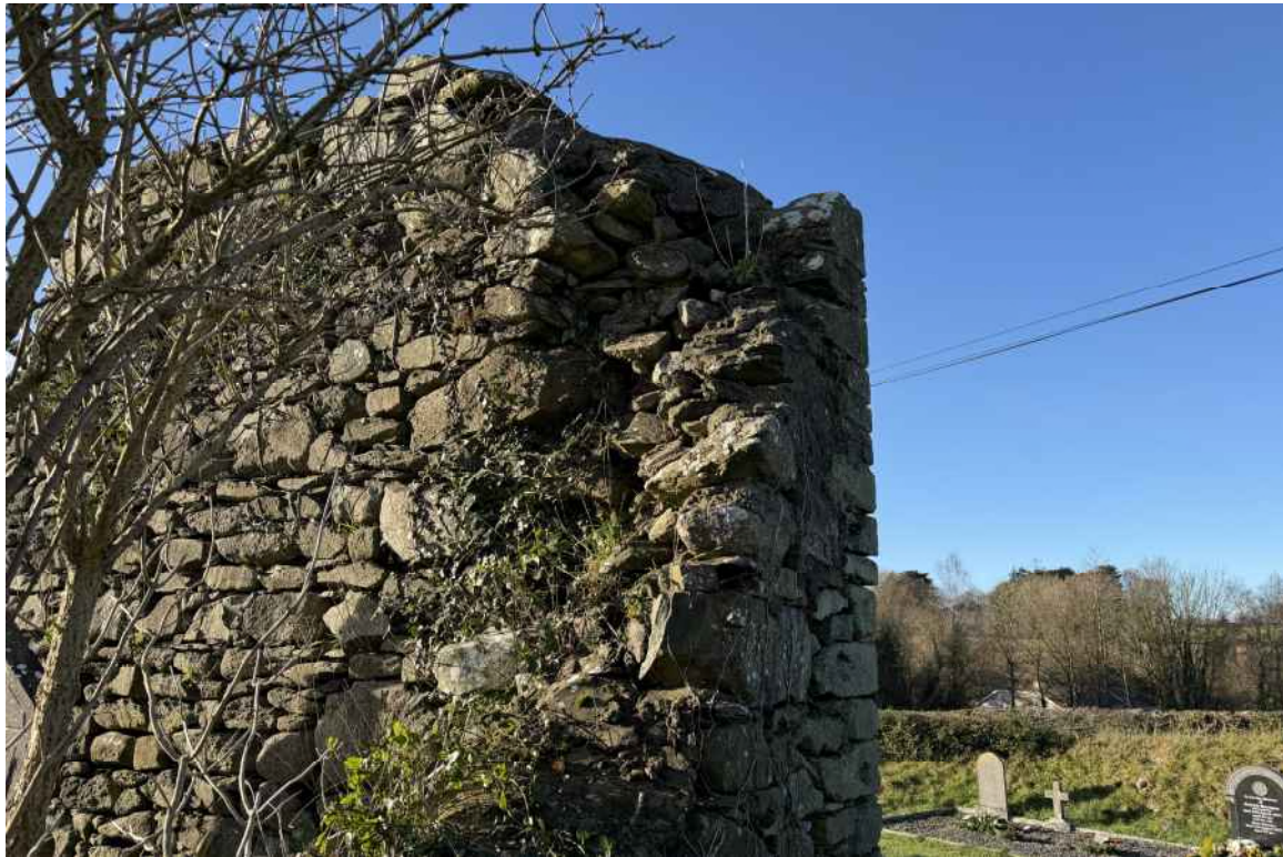
PHOTOGRAPH 11 - EXPOSED CORE AT THE NORTHWEST CORNER
