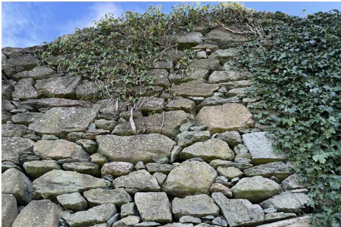
PHOTOGRAPH 4 - IVY STEMS GROWING FROM CORE OF THE WALL AT THE WEST GABLE
