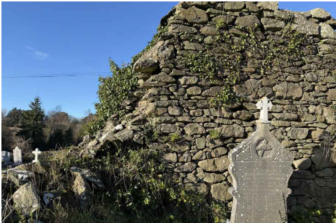
PHOTOGRAPH 12 - LOOSE MASONRY AT SOUTH VERGE OF WEST GABLE
