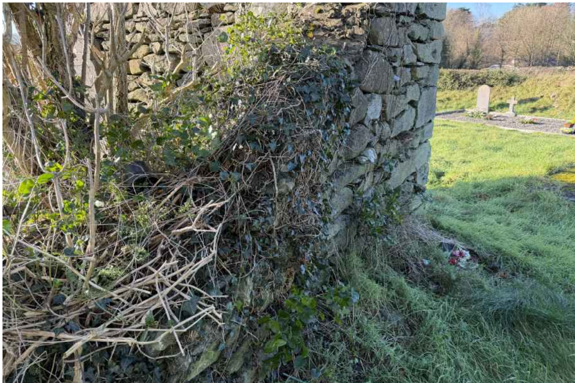
PHOTOGRAPH 8 - DISLODGED MASONRY AT THE NORTH WALL RETURN
