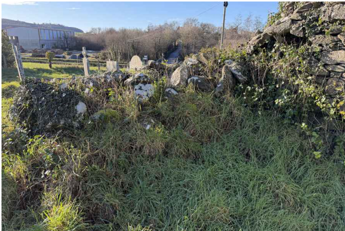
PHOTOGRAPH 13 - REMAINS OF SOUTH WALL INNERFACE AT WEST GABLE
